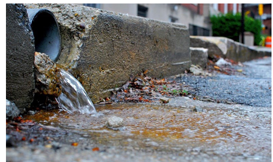
On-site property drainage is key to improving community challenges with stormwater. (Source: Township of Susquehanna)
