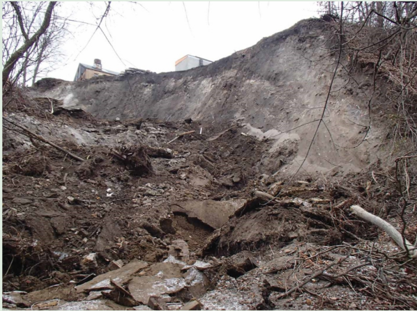
The slope after the landslide
