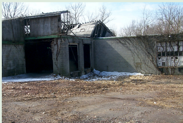
Derelict Plating Facility Before DEP Cleanup
