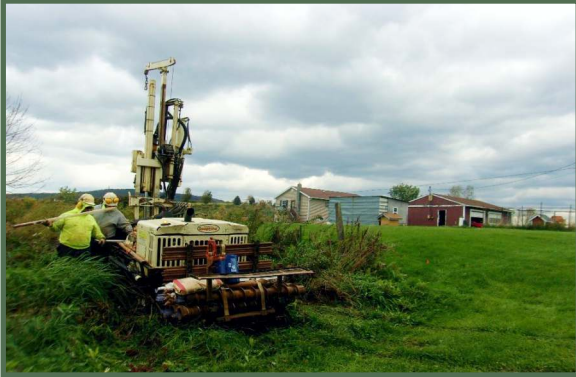
Direct push borings were advanced for soil characterization and piezometer installation in strategic locations.
