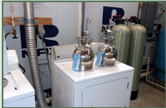
Air sampling was conducted at the impacted home to ensure that the vapor mitigation system was effective in removing TCE from the ambient air.
