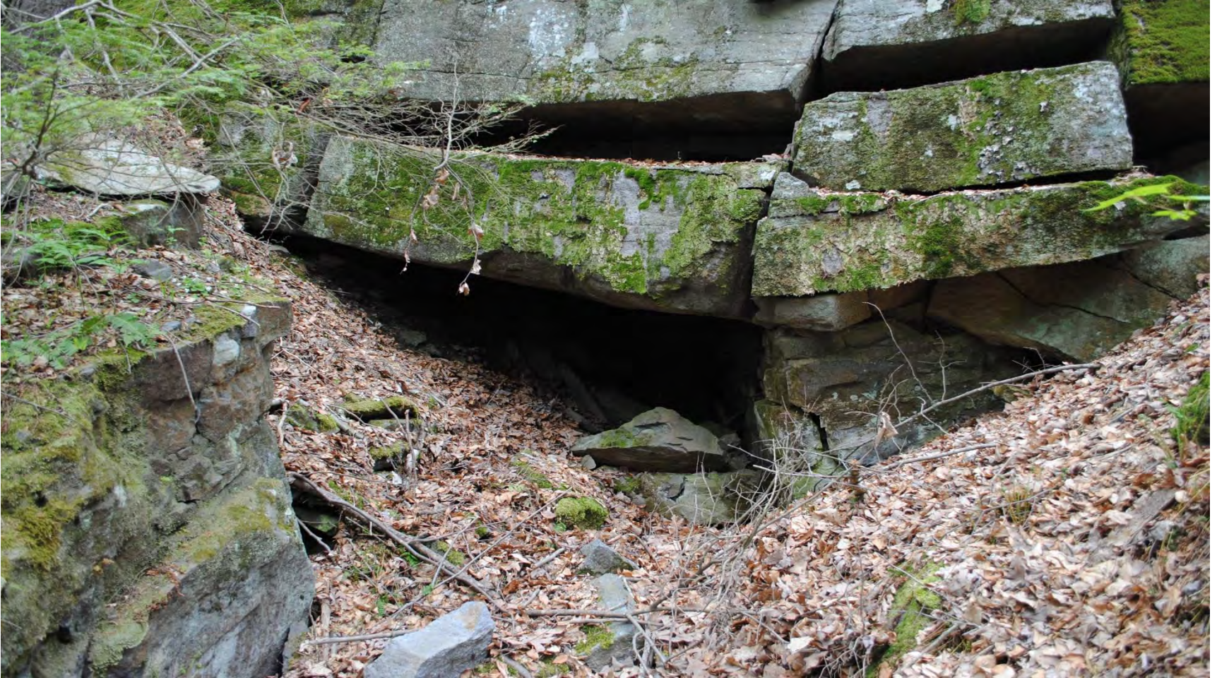
Feature 2157-06 Mine Opening
