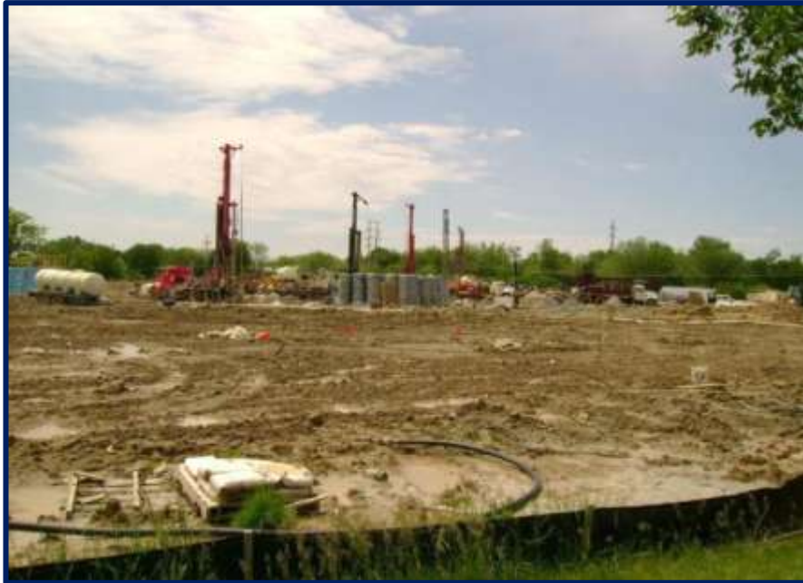
Photo shows drill rigs at Ball State boring a portion of what will be some 3600 wells buried under an old soccer field, parking lots and 25-40 acres of green fields.
