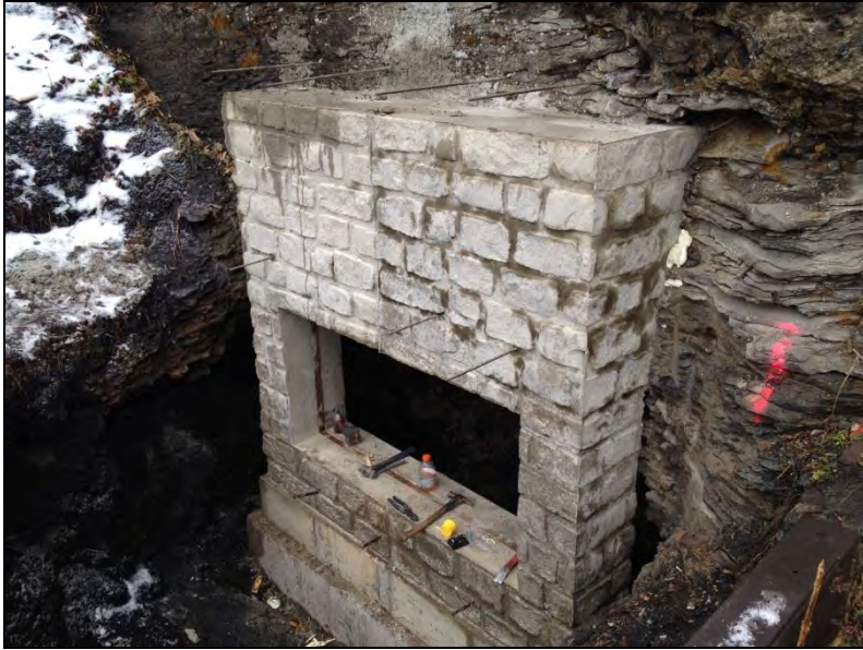
Poured concrete bat gate prior to staining and installation of angle iron.
