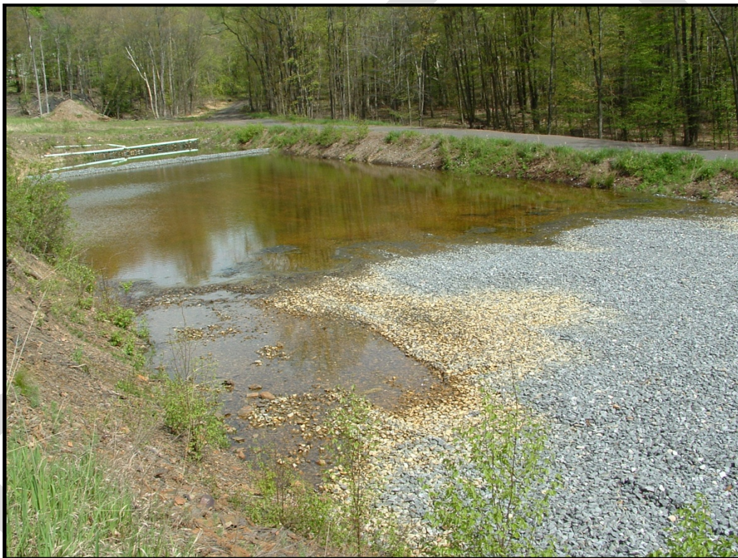
Figure 7.13. Water pooling indicates plugged sections of a RLB
