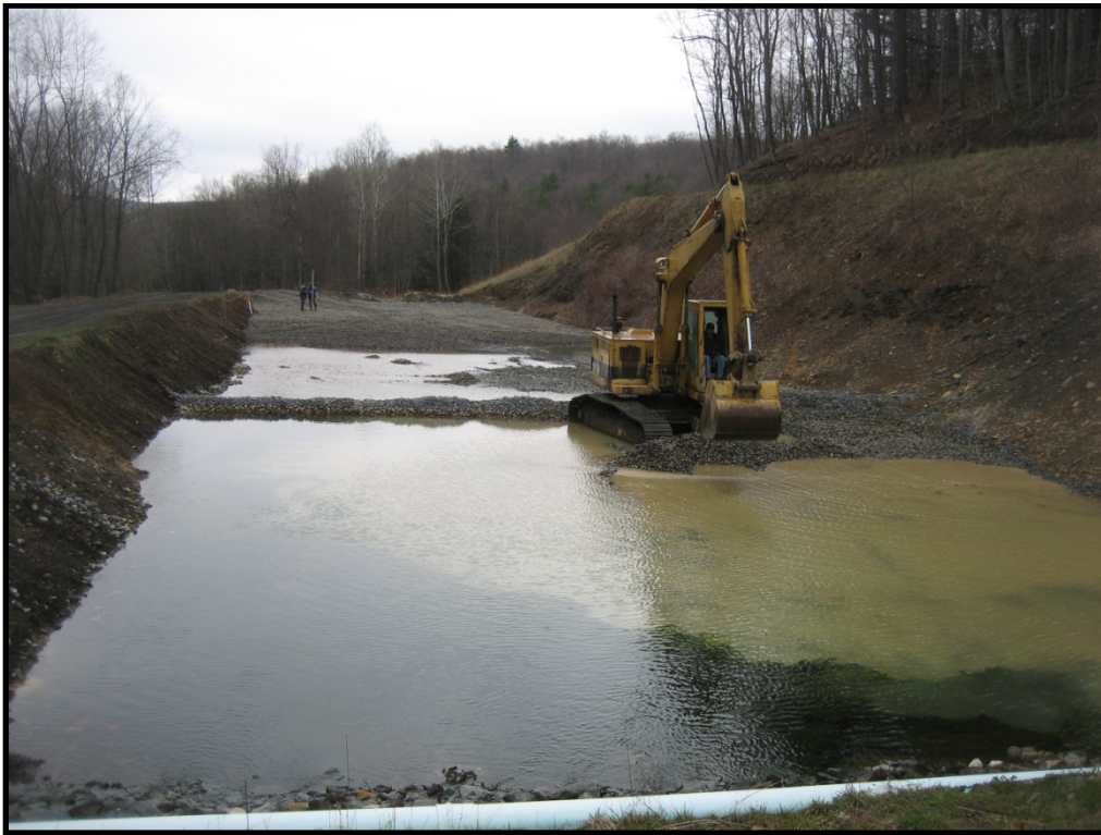
Figure 7.14. Agitation using an excavator to break up precipitate and reestablish flow in a clogged section of a RLB
