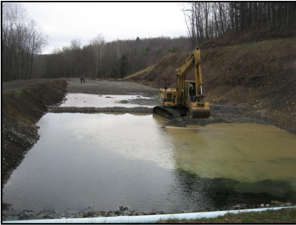
Figure 7.14. Agitation using an excavator to break up precipitate and reestablish flow in a clogged section of a RLB
