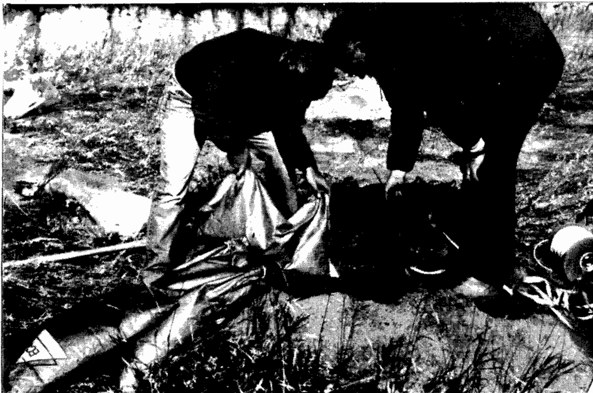
FIGURE 5-4: THE LOADING OF ANFO INTO A BLASTHOLE WITH THE BLASTING TAPE BEING USED TO MONITOR THE COLUMN RISE
