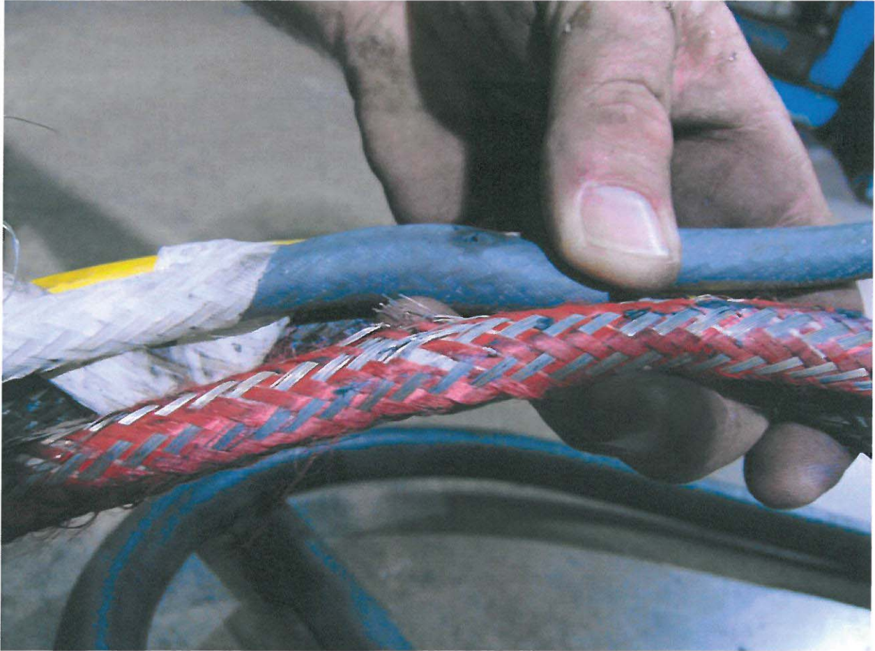
SHDGC shield wires penetrated the insulation causing the trip.
