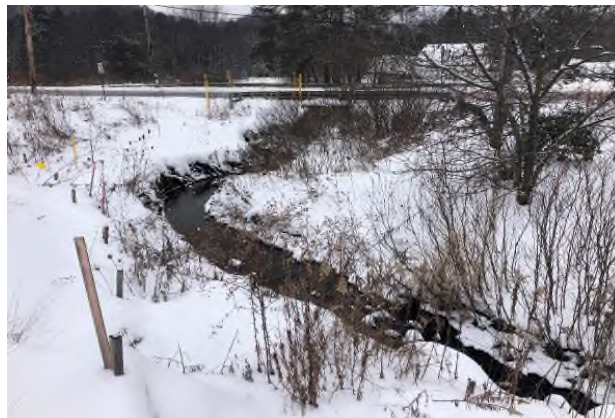
Photo # 27 : 01/27/2019 -- Stream 044 UNT to Hinckston Run (CWF) Facing west or downstream along O44 on the eastern side of William Penn Ave (SR-271). Compost filter sock installed along stream channel is unrelated to Mariner East II project.
