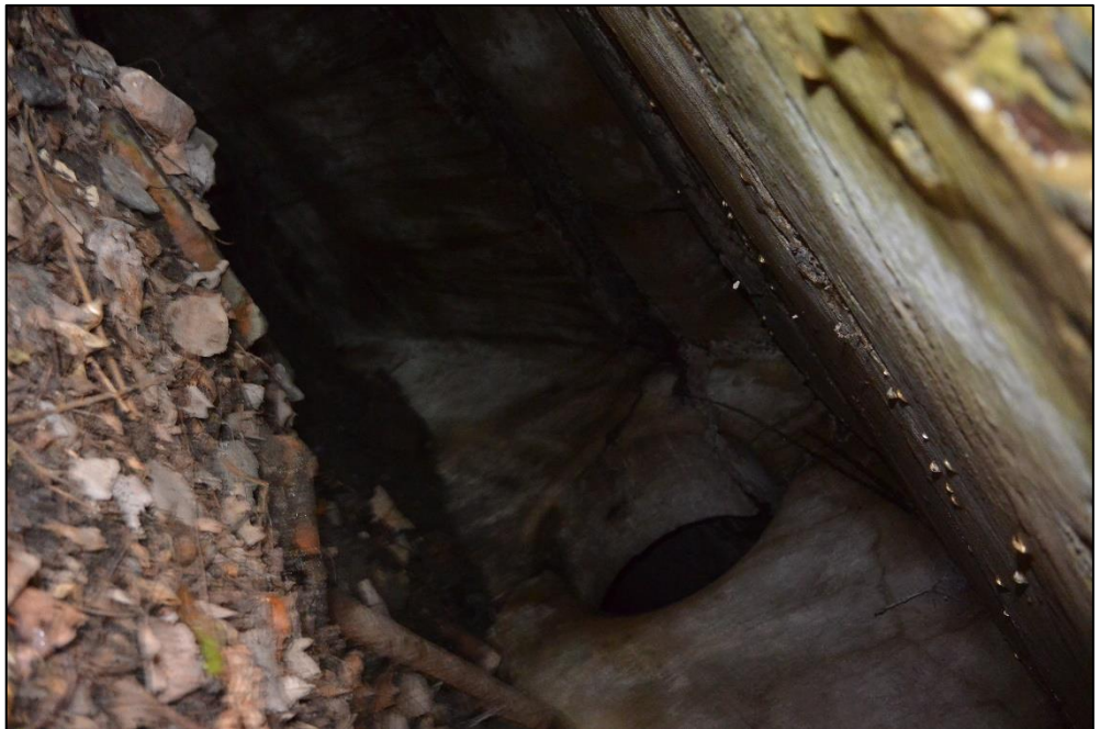
Figure 11: RedAsh Shaft, photograph within void of Figure 10, showing concrete structure below surface debris. April 2016
