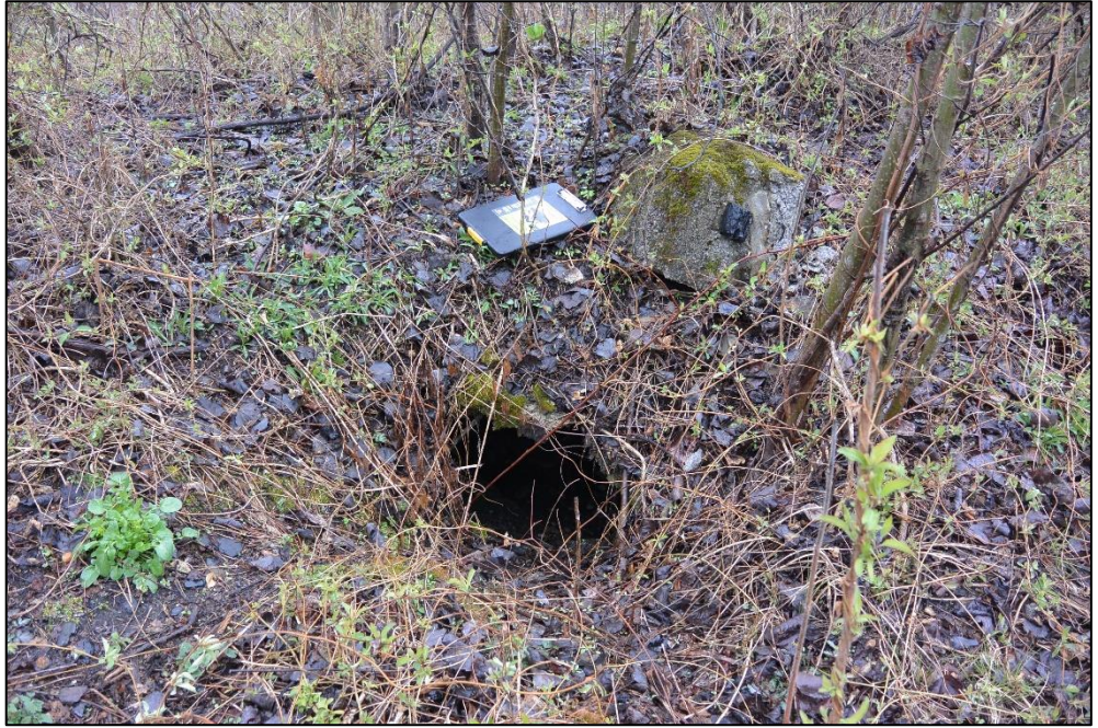
Figure 10: RedAsh Shaft, void in mounded shaft area. April 2016
