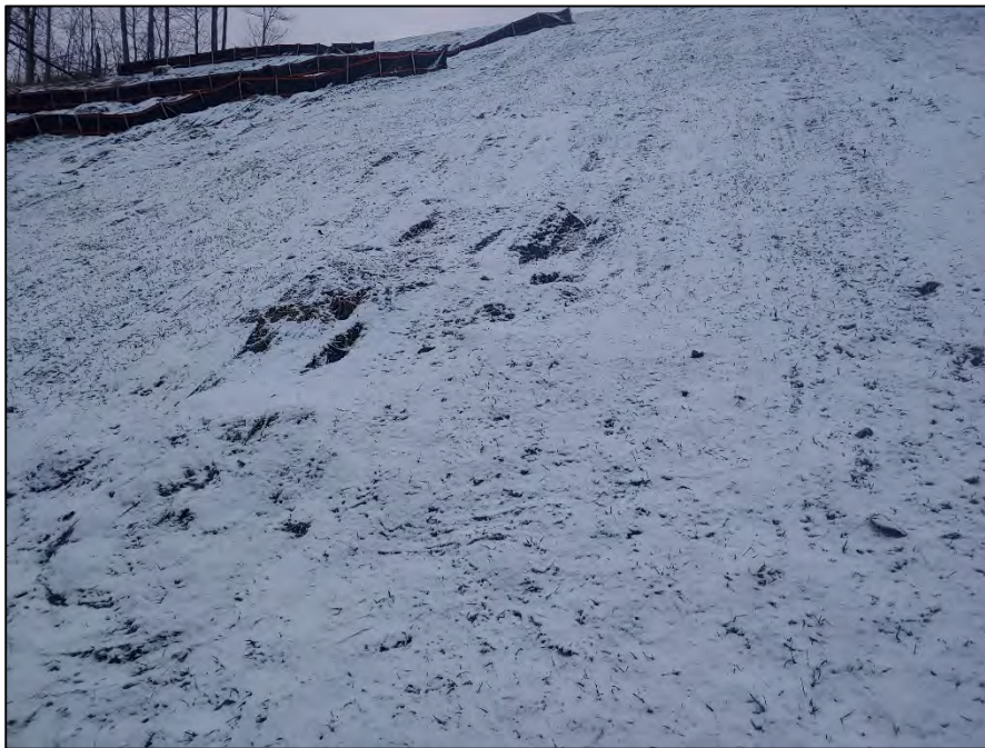
Looking upslope at the slope failure near station 1351+00
