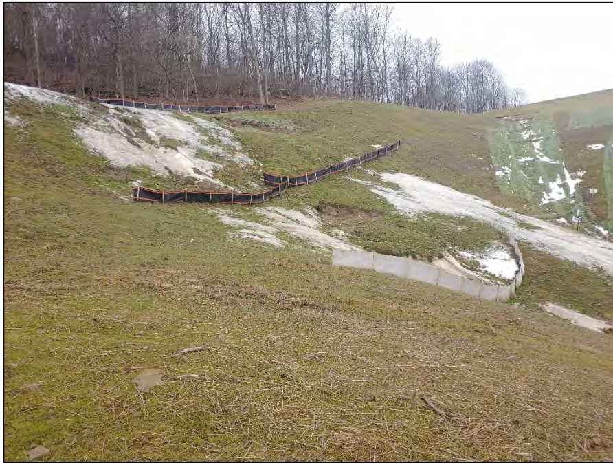
Looking west towards the slump material at Elkhorn Run 2 near station 872+00
