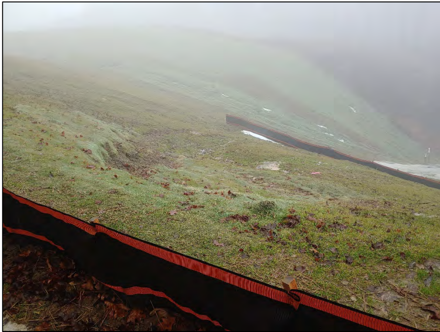
Looking north towards the slump material at Elkhorn Run 2 near station 872+00
