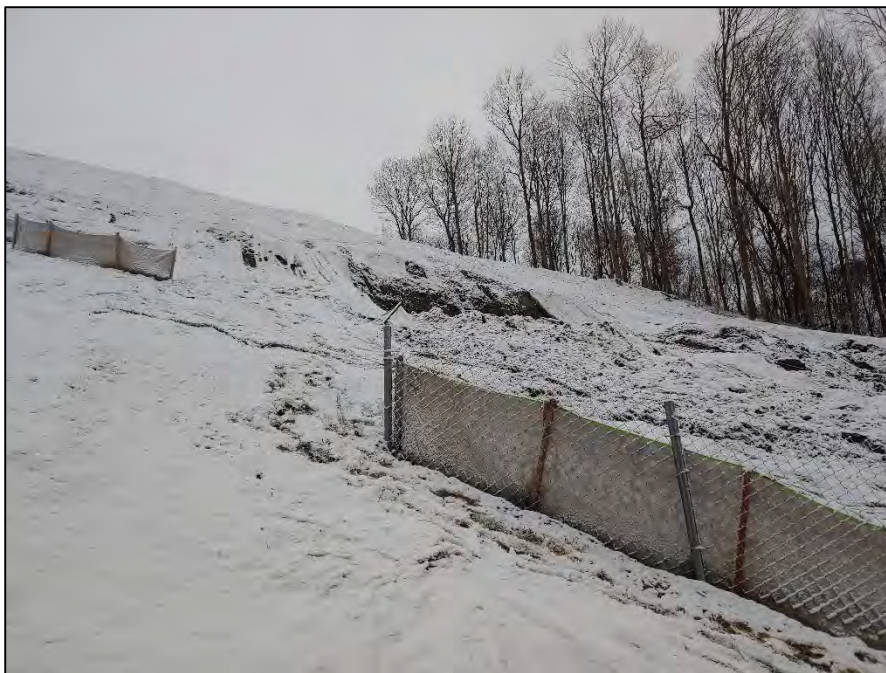
Looking west at the landslide near station 1173+00
