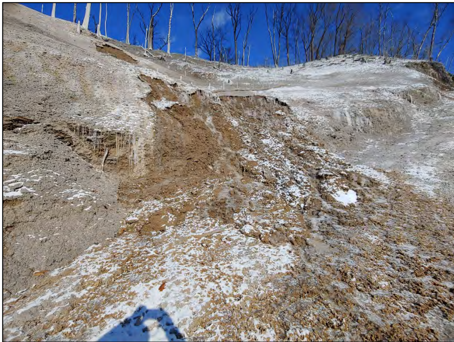
Looking upslope at the shallow landslide near station 1115+50
