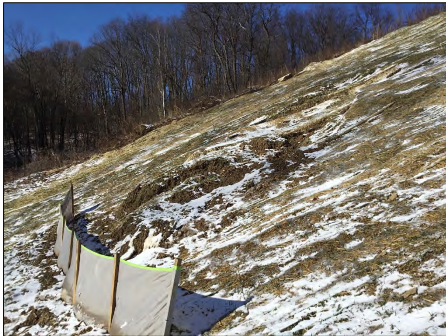
Looking west at the shallow surface slump near station 962+50
