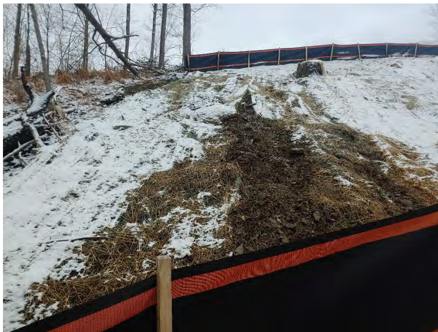
Looking upslope at the slope failure near station 1353+00
