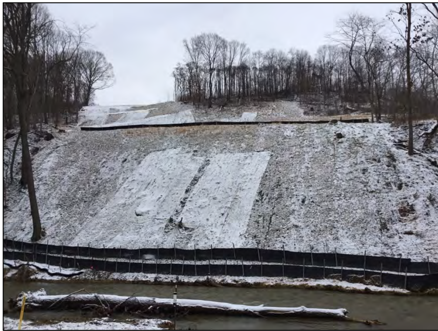
Looking east towards the surface failure near station 789+00
