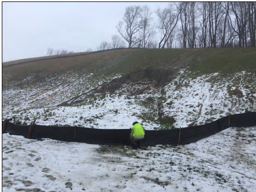
Fill failure near station 734+50
