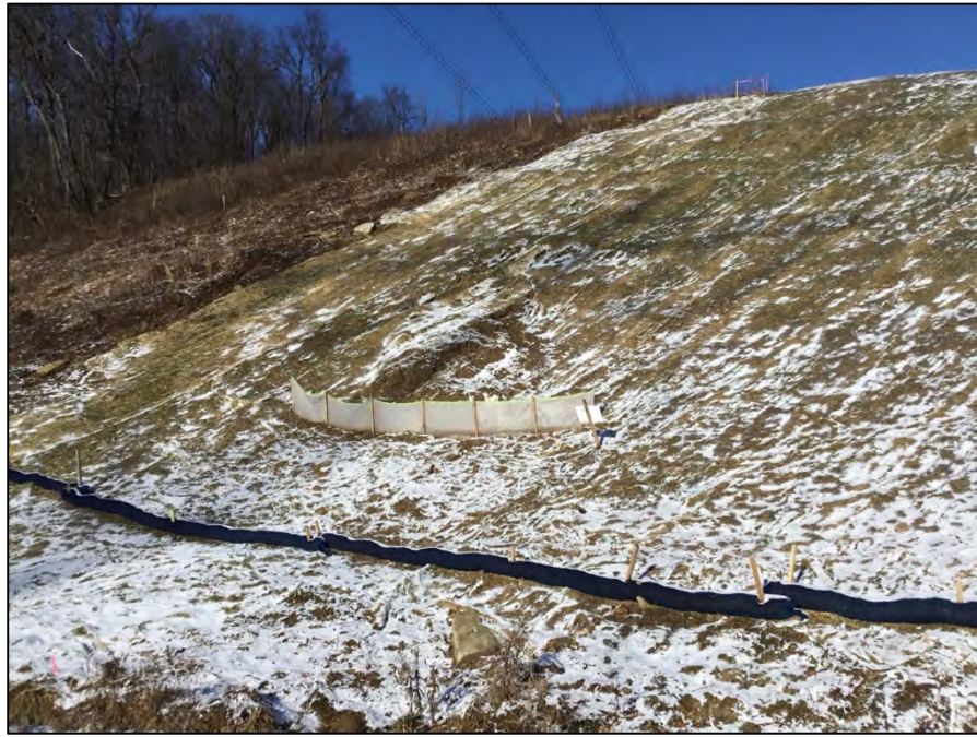
Looking northwest at the shallow surface slump near station 962+50
