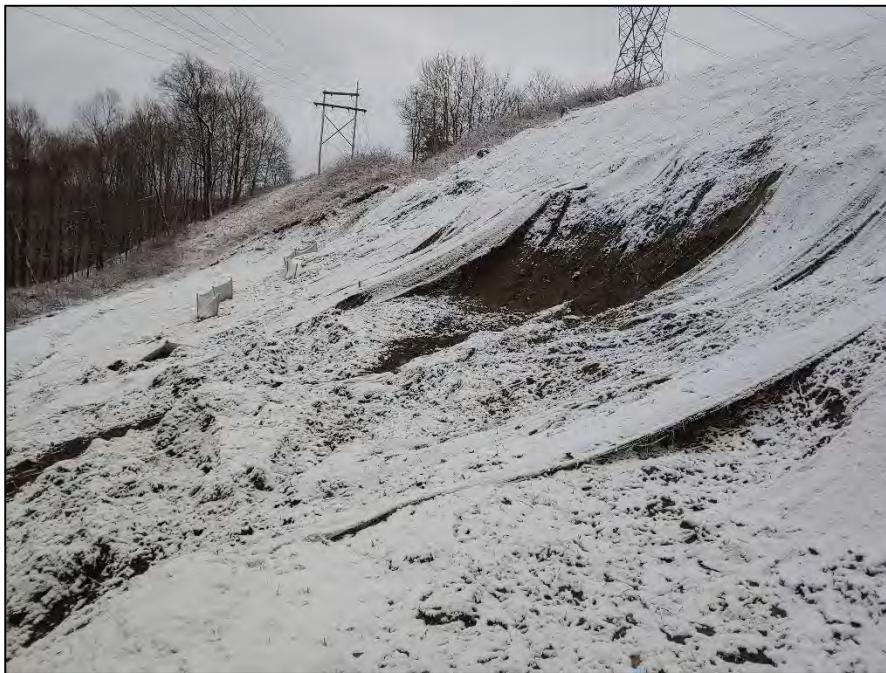
Looking south at the landslide near station 1173+00
