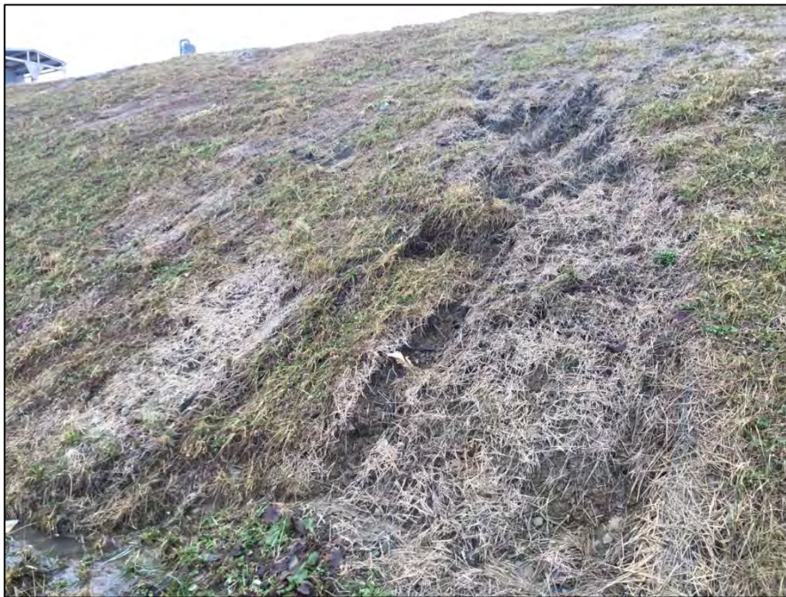
Looking south at the surface slump near station 2151+50
