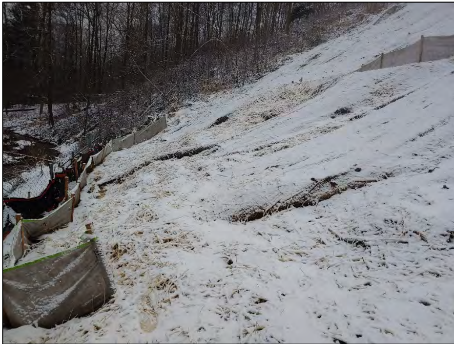
Looking at the landslide near station 1313+00
