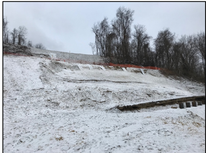
Looking northwest at reggraded landslide below Penny Hollow Road and H-piles installed at toe.
