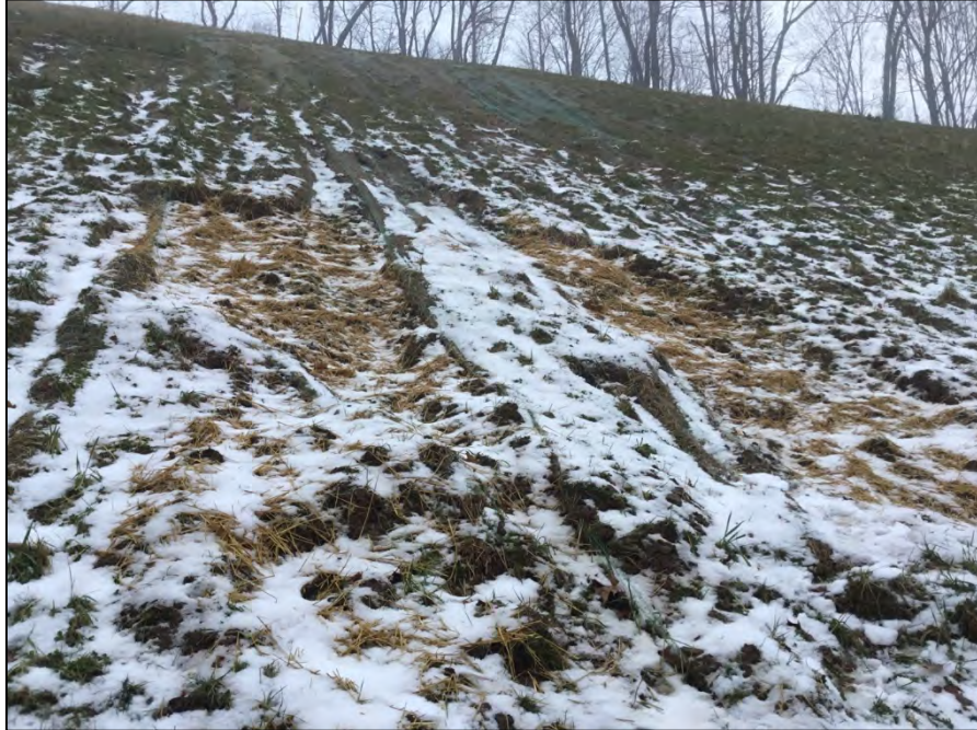
Shallow surface raveling near station 735+50
