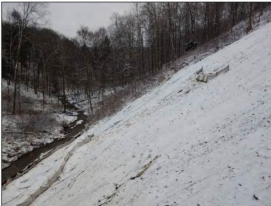
Looking at the landslide near station 1313+00
