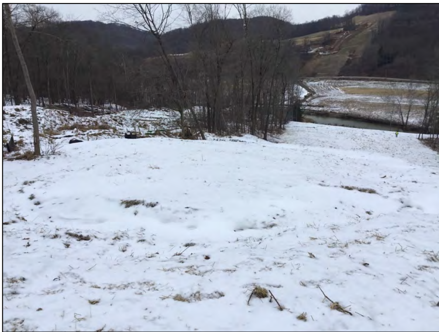
Looking north at the landslide near station 1632+00
