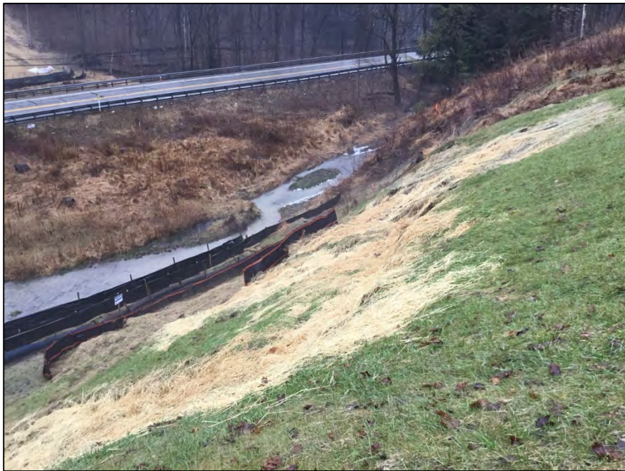
Looking east toward the surface failure near station 1698+00
