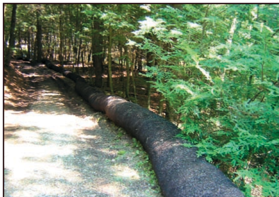
24 in Runoff Diversion for High Storm Flow
