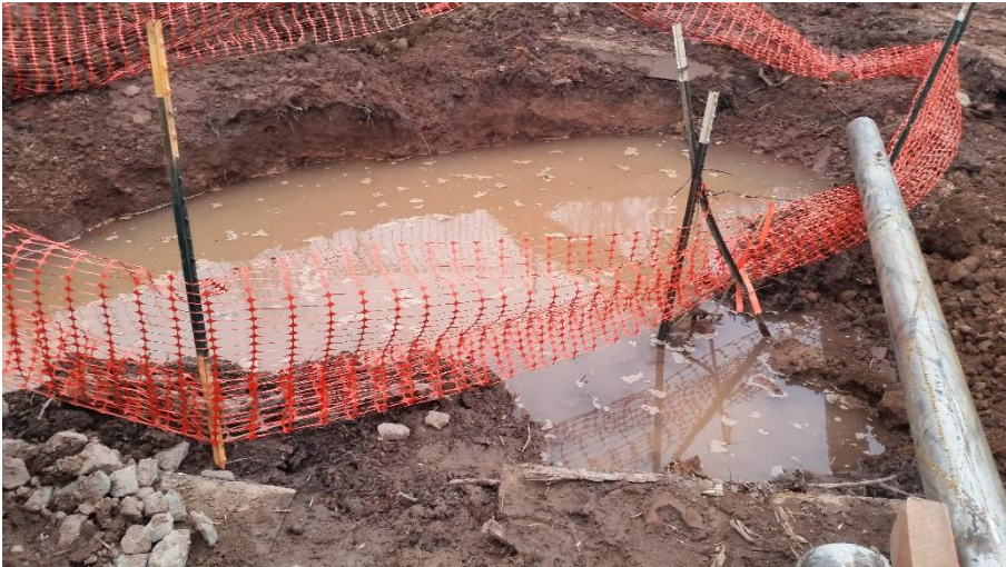
Drill pit constantly fills with ground water, West side of HDD alignment.
