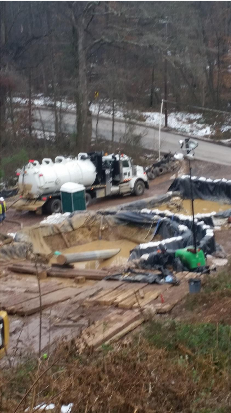
November 19, 2018 Pipe is pulled through, both containment areas are full flooded with drilling mud.
