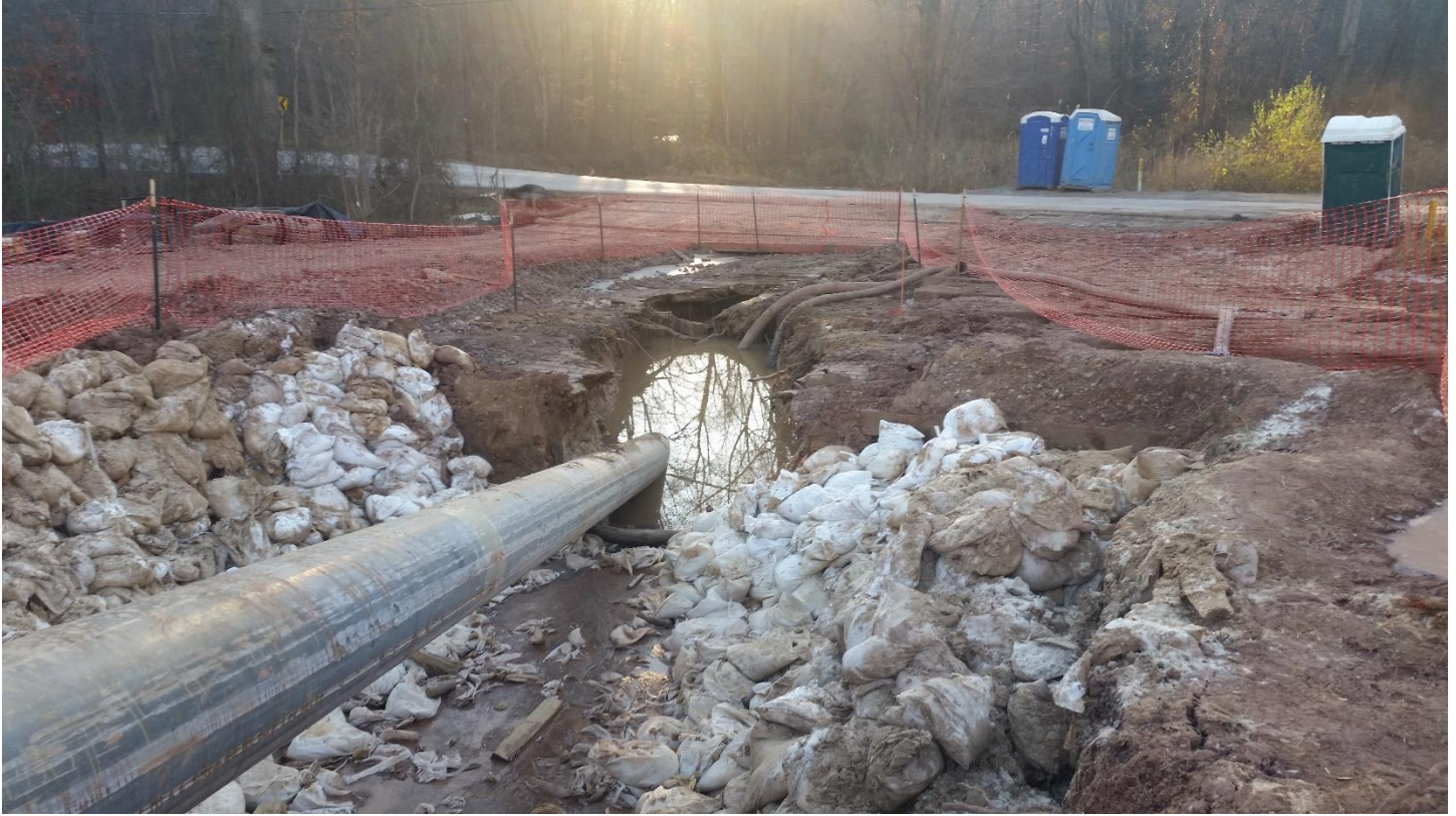
November 24-24, 2018 Additional removal of timber mats is conducted revealing the extent of undermined soils. Drill pit extends nearly to the road, vac truck runs continually to keep pit dry for welding.
