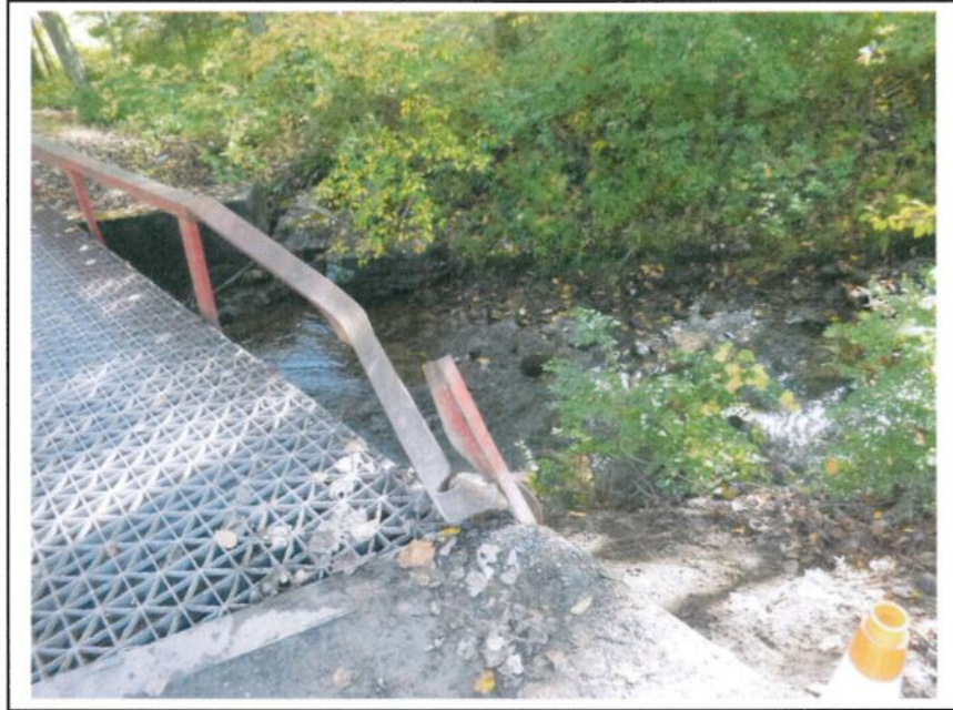
Photo No. 17: Near Right Railing Damage
