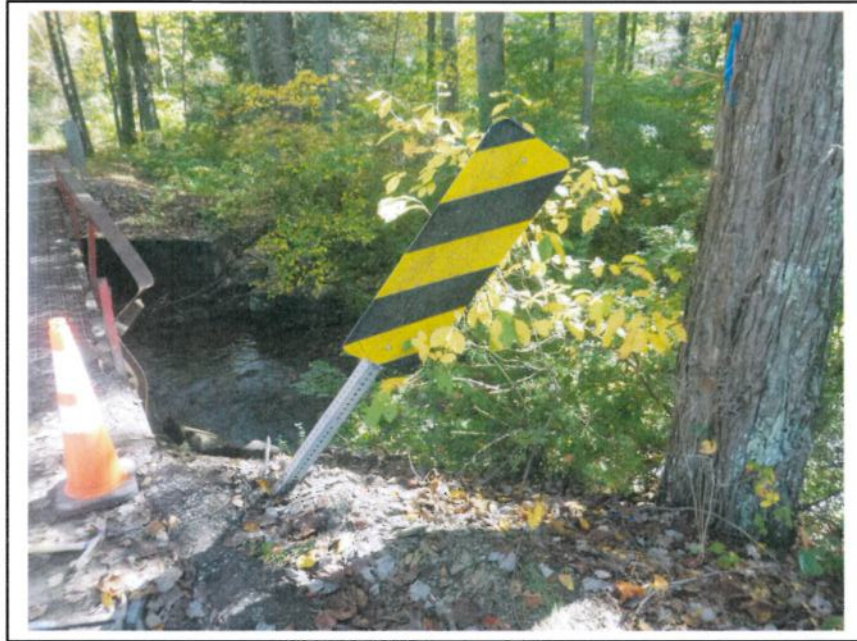
Photo No. 15: Near Right Leaning Hazard Clearance Sign
