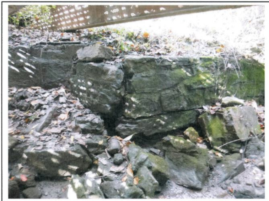
Photo No. 32: Near Left Abutment Voids
