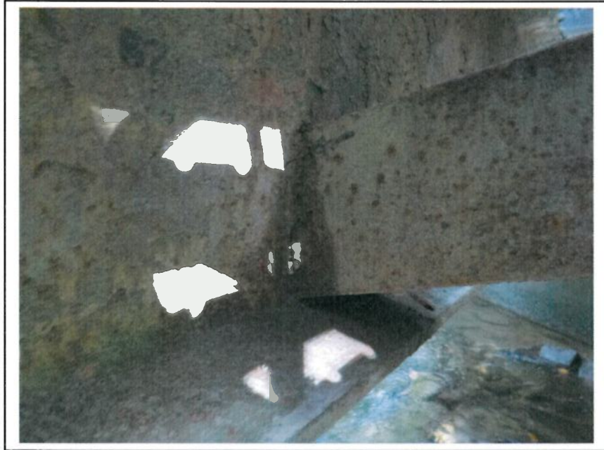
Photo No. 29: Bay 2 Cracked Weld at Beam 2
