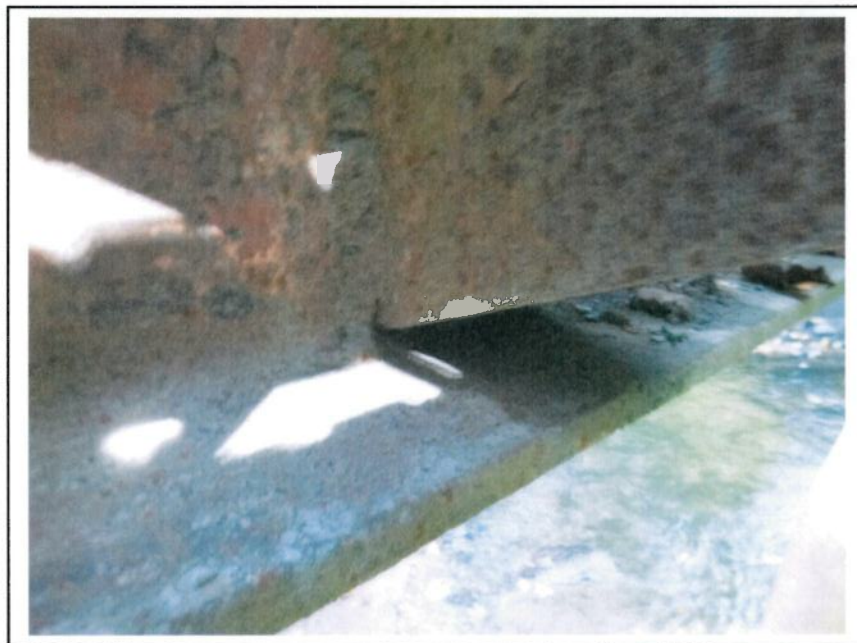
Photo No. 28: Bay 1 Intermediate Diaphragm Cracked Weld at Beam 1
