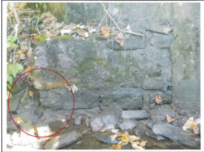
Photo No. 37: Far Left Wing Void
