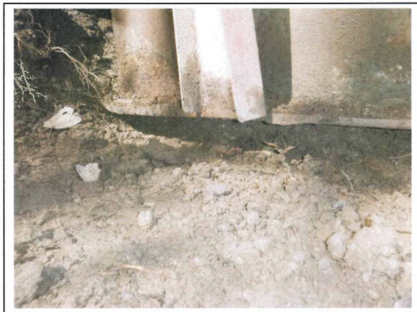
Photo No. 26: Beam 4 Loss of Bearing at Near Abutment
