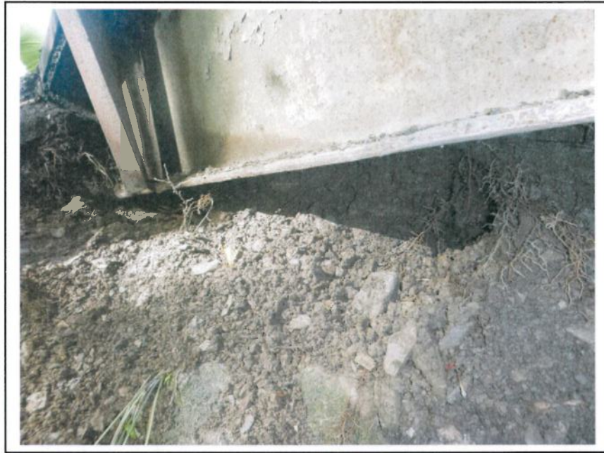
Photo No. 25: Beam 4 Loss of Bearing at Near Abutment
