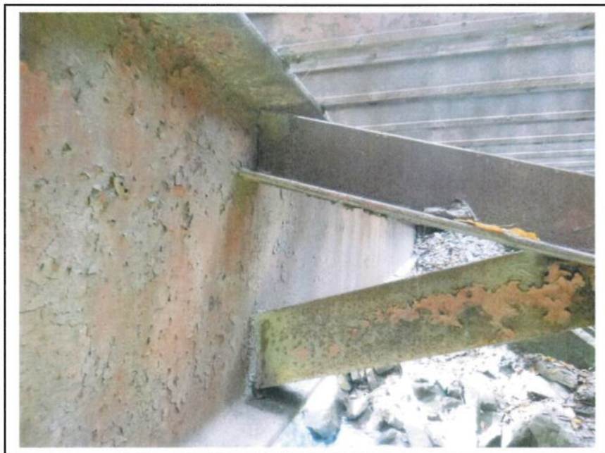
Photo No. 30: Bay 3 Intermediate Diaphragm Gap in Connection
