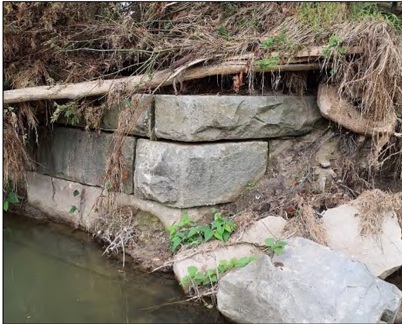
5. View of the stone bridge abutment that carried the former New York Central and Hudson River Railroad over the Cowanesque River. Facing southwest.
