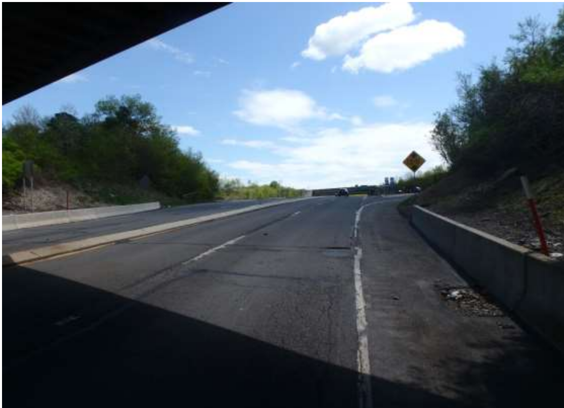
Direction / Road: SB Route 54 (Vulcan Hill Rd) Approach / Departure: Approach Distance: 200 feet
