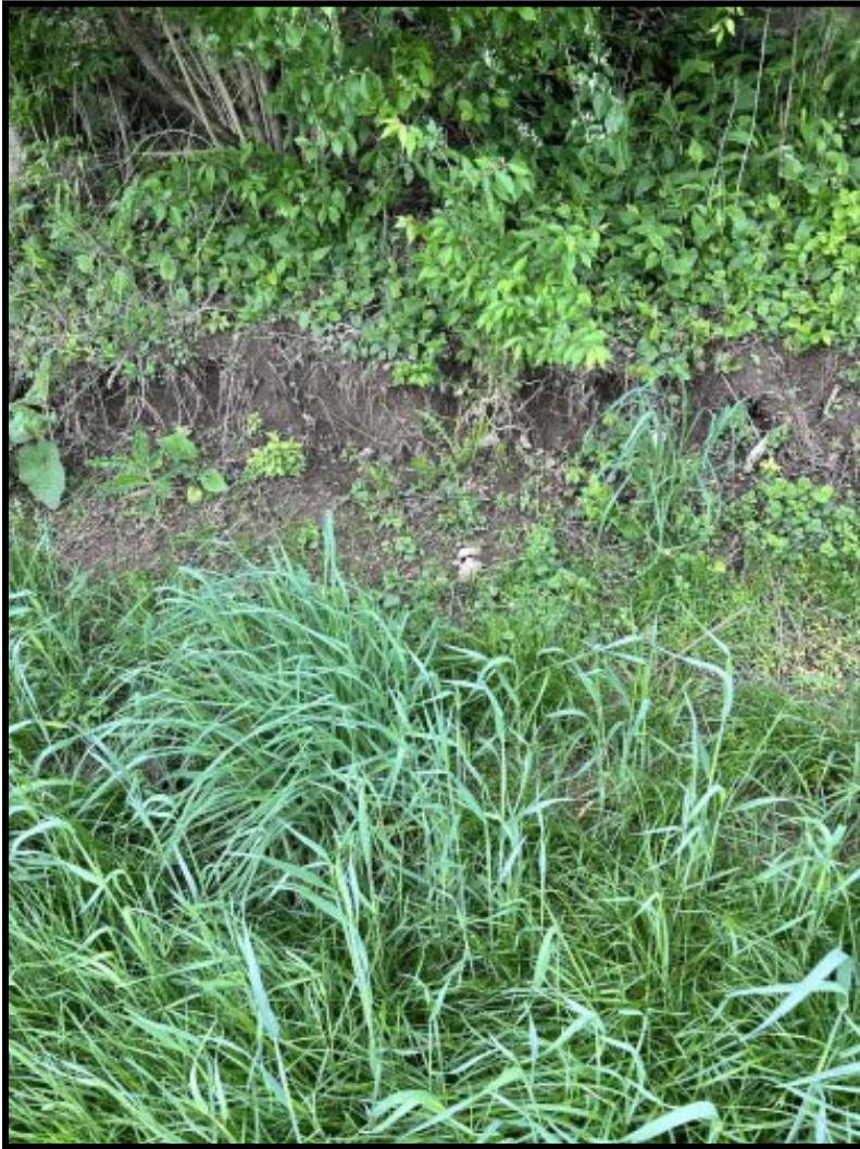
Photograph 15 – Sloughing observed upslope of sag topography at approximate Station 160+00.
