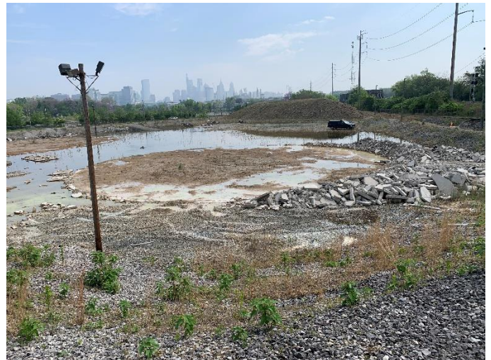
TK-7550 / TK-7551 tank containment with discoloration
