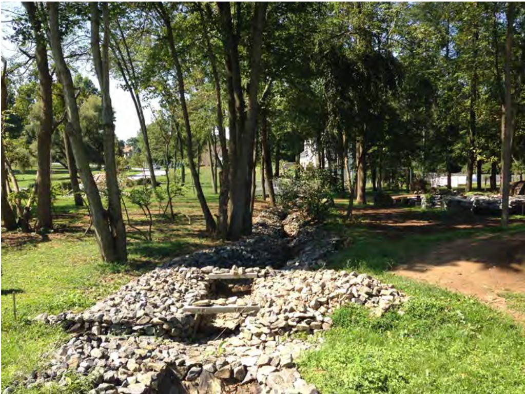
38. View west of a rip-rap channel (S-B34) within the ROW of the pipeline within Parcel PA-DE-0008.0000 (September 4, 2014).
