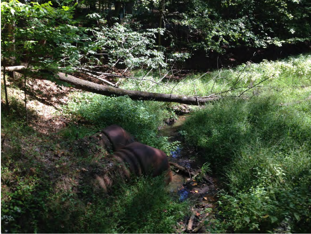
69. View of a forested stream channel (S-I12) and outfall pipes associated with abandoned stormwater management ponds within Parcel PA- DE-0150.0000 (September 12, 2014).
