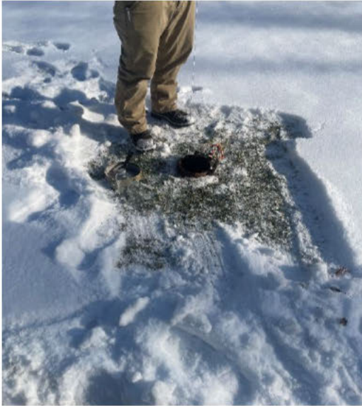
Photo 1 Open well head
