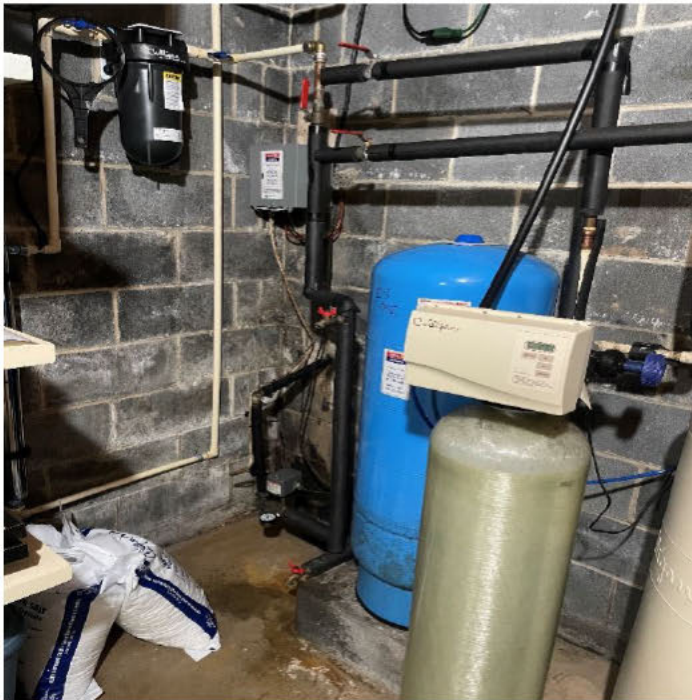
Photo 3 Basement treatment system
