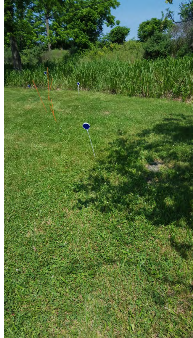
Figure 2 Suspected Sinkhole Area Looking Northwest from Phillips Mill Road
