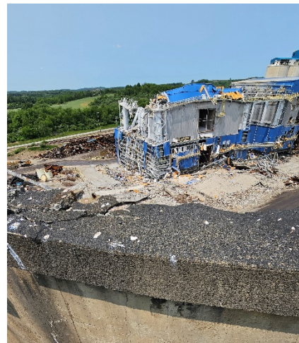
Photo 30: UNIT #3 TOP ASH SILO NO VISIBLE ACMS
