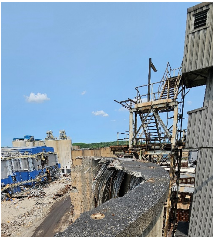
Photo 29: UNIT #3 TOP ASH SILO NO VISIBLE ACMS
