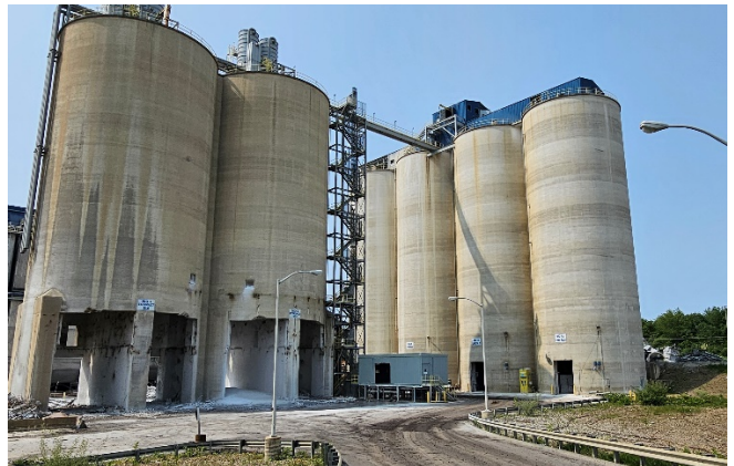
Photo 12: LIME AND BYPRODUCT SILOS
