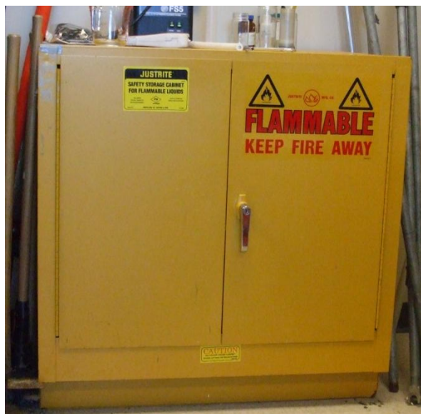
FLAMMABLE STORAGE CABINET
