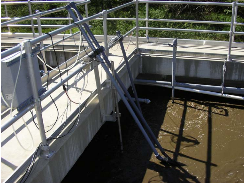
Figure 35: Nitrate, Ammonium, TSS and pH probes installed in South aeration tank
