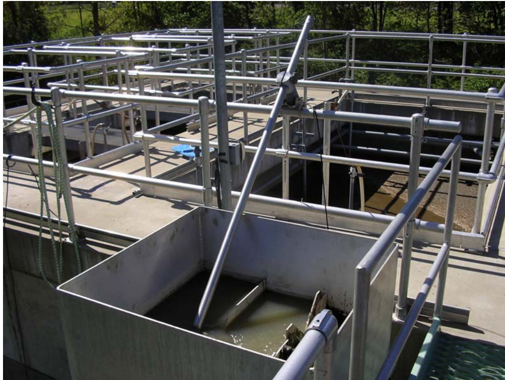
Figure 39: UVAS probe mounted at influent splitter box
