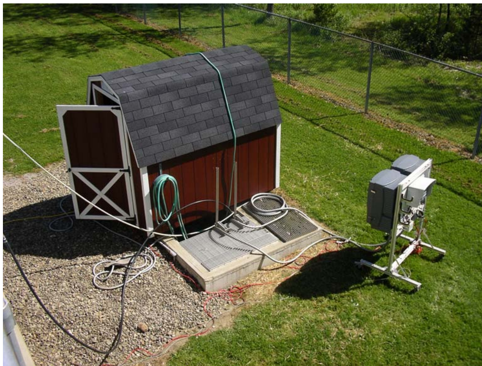
Figure 40: Amtax and Phosphax probes mounted at the chlorine contact
