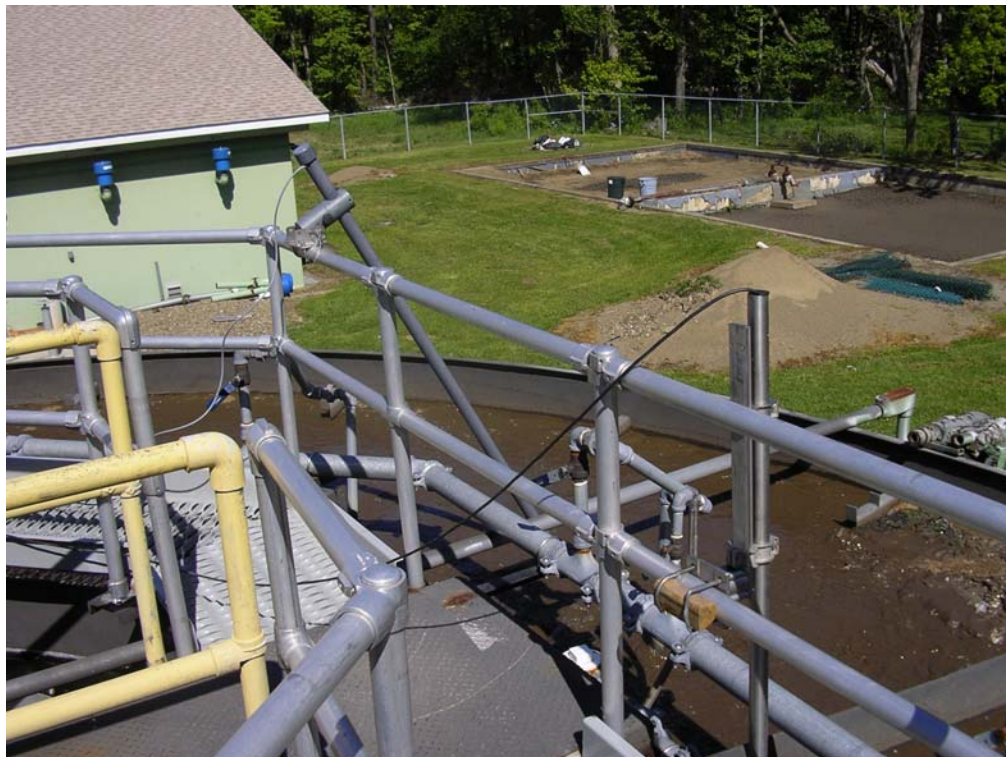
Figure 38: TSS probe mounted in North aeration tank
