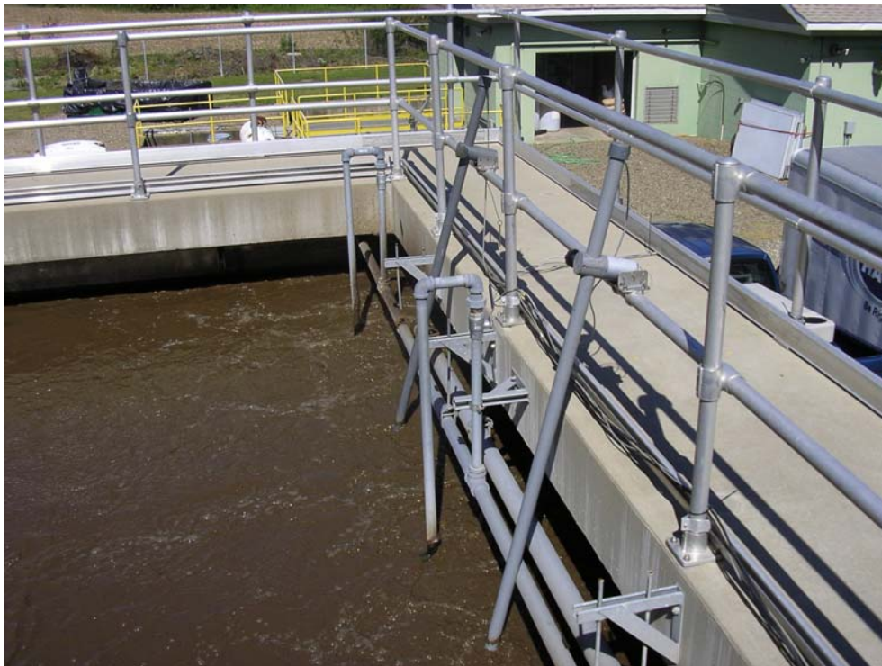
Figure 36: LDO and ORP probes installed in South aeration tank
