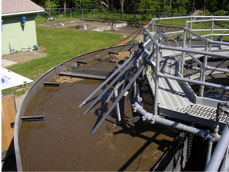
Figure 37: Nitrate, Ammonium, pH, LDO, and ORP probes installed in North aeration tank
