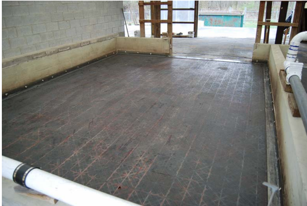
Figure 44. Solids drying bed number 2
