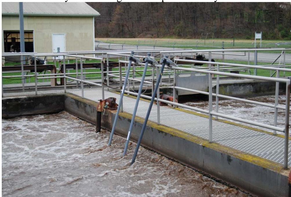
Figure 42. DO, ORP, and pH probes installed in south aeration tank
