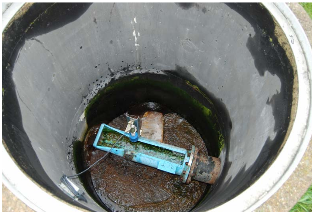
Figure 47. Effluent metering pit just prior to stream discharge
