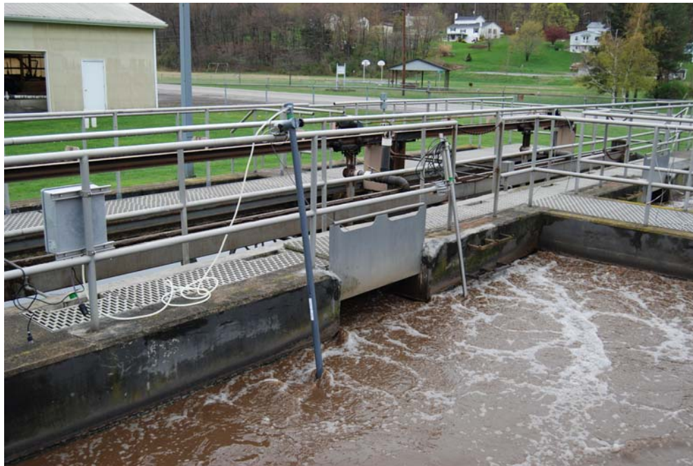
Figure 43. Nitrate and NH 4 D probes installed in south aeration tank
