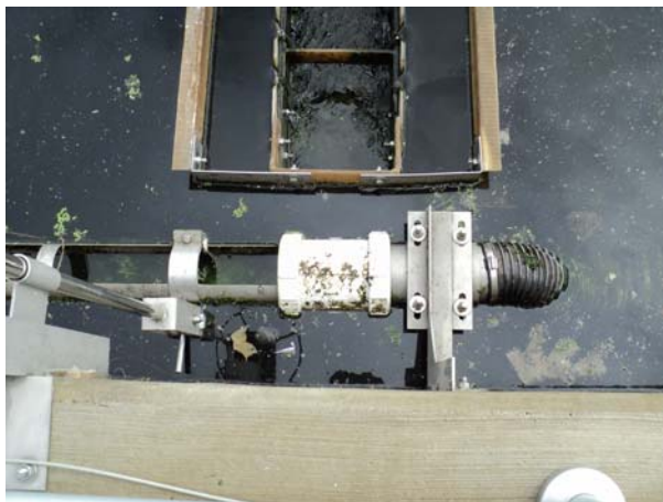
Figure 3.10 Surface skimmer coupling in west clarifier
