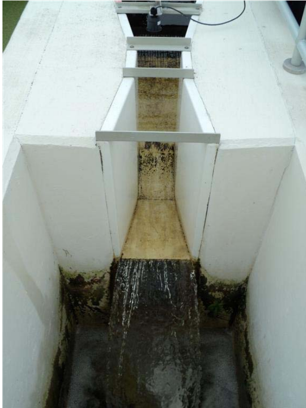
Figure 3.13 Chlorine contact tank discharge
