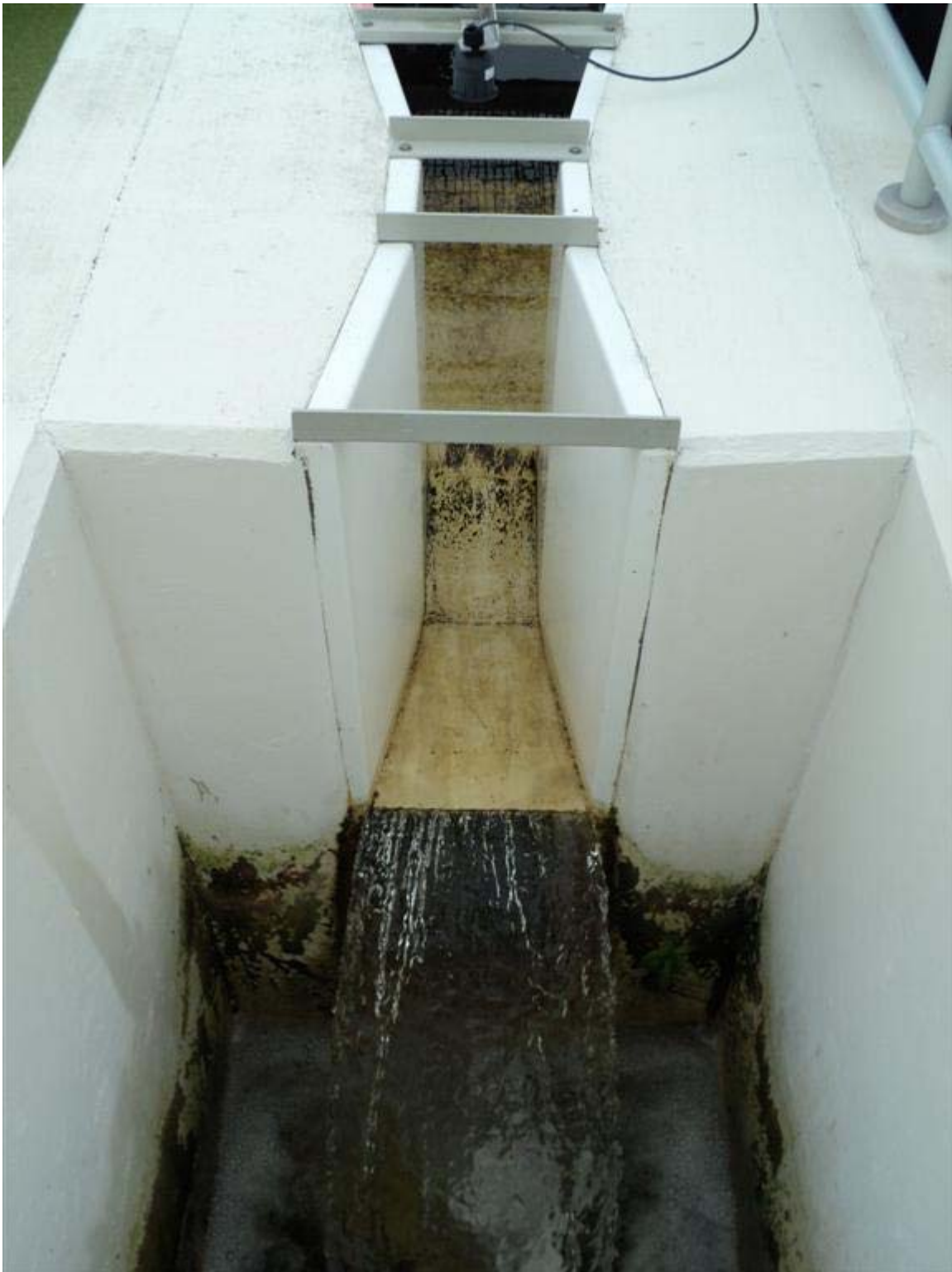
Figure J.5 Chlorine contact tank discharge
