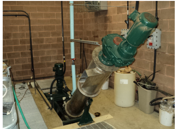
Figure 3.2 Elkland headworks auger system
