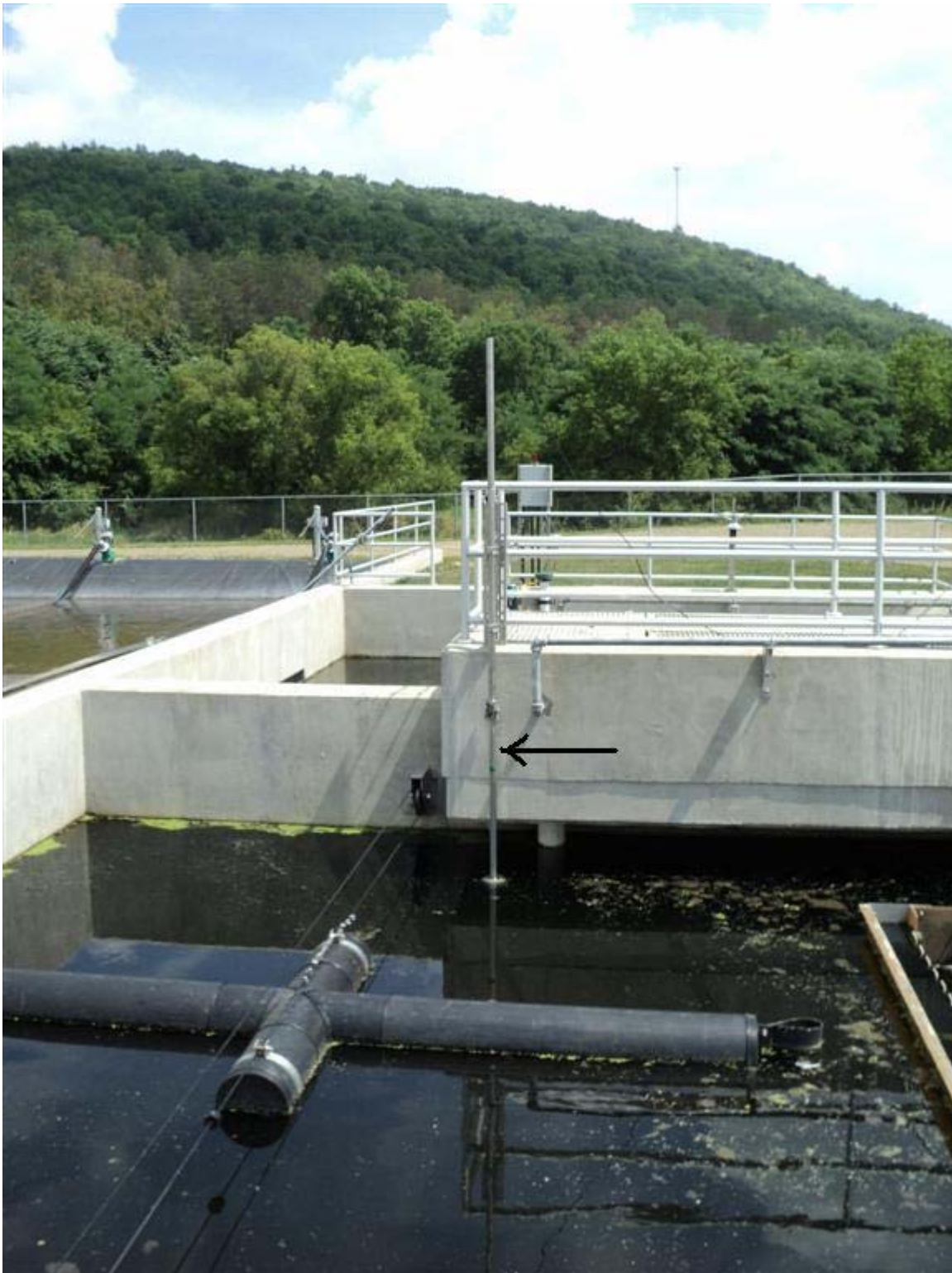
Figure J.2 Sonatex probe installed in west clarifier
