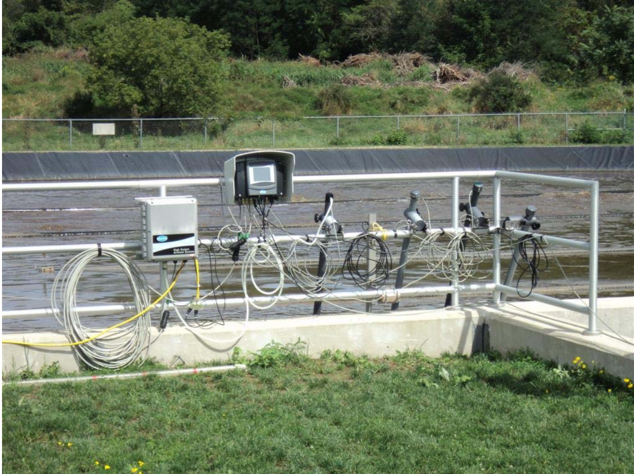
Figure J.1 DO, ORP, Ammonium, Nitrate, and TSS probes installed in north lagoon 1A
