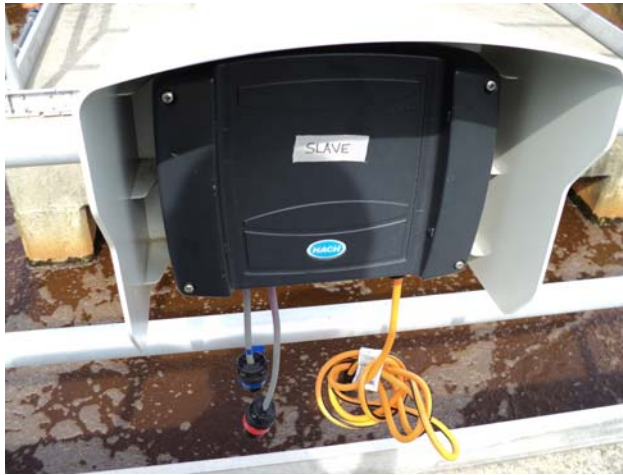
Figure F.1: SC-1000 Base Unit, Stage 2 Aeration
