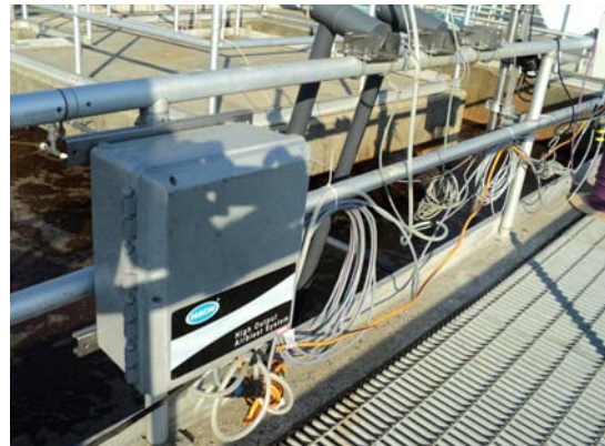
Figure F.4: Stage 2 Air Compressor in Operational Mode
