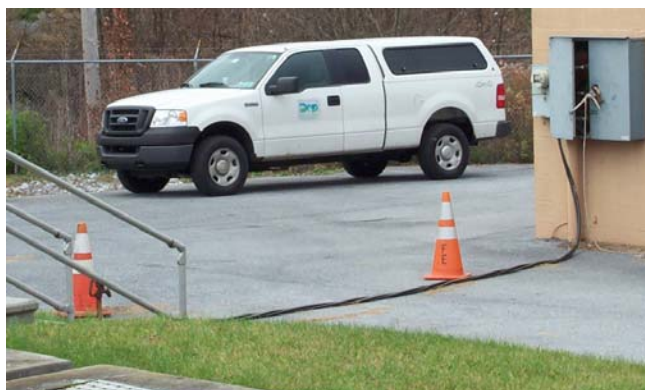
Figure: Temporary main power line from transformer on pole.
