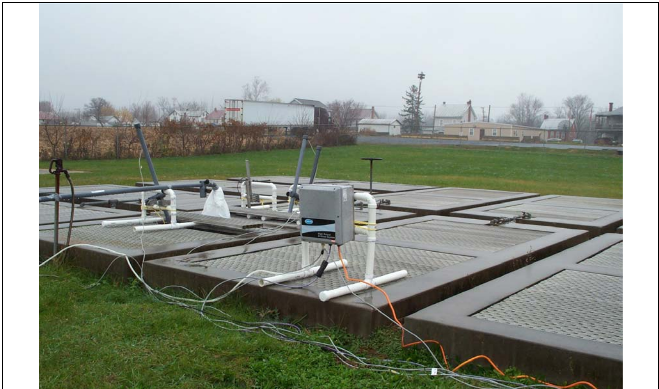
Figure F-3: Air compressor (center) for Ammonia probe cleaning system, on mounts.
