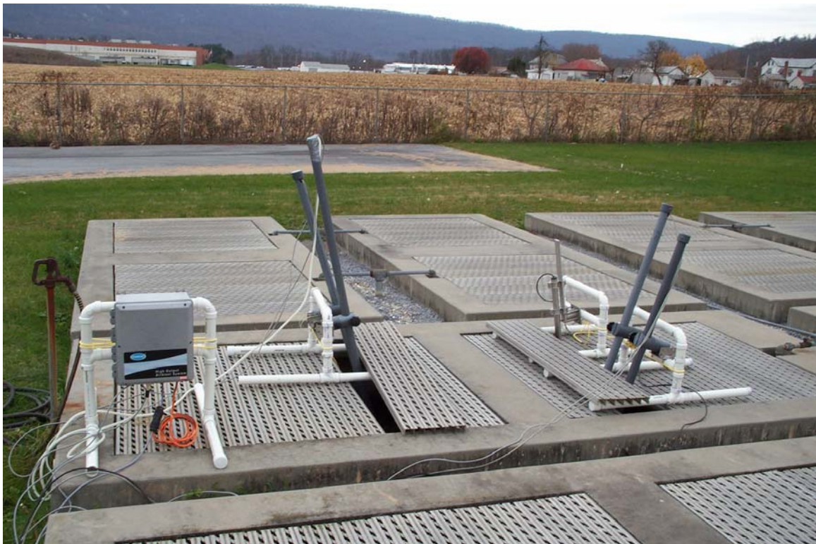
Figure F-6: Sensor Probes set up in Tank 6 of west aeration train.
