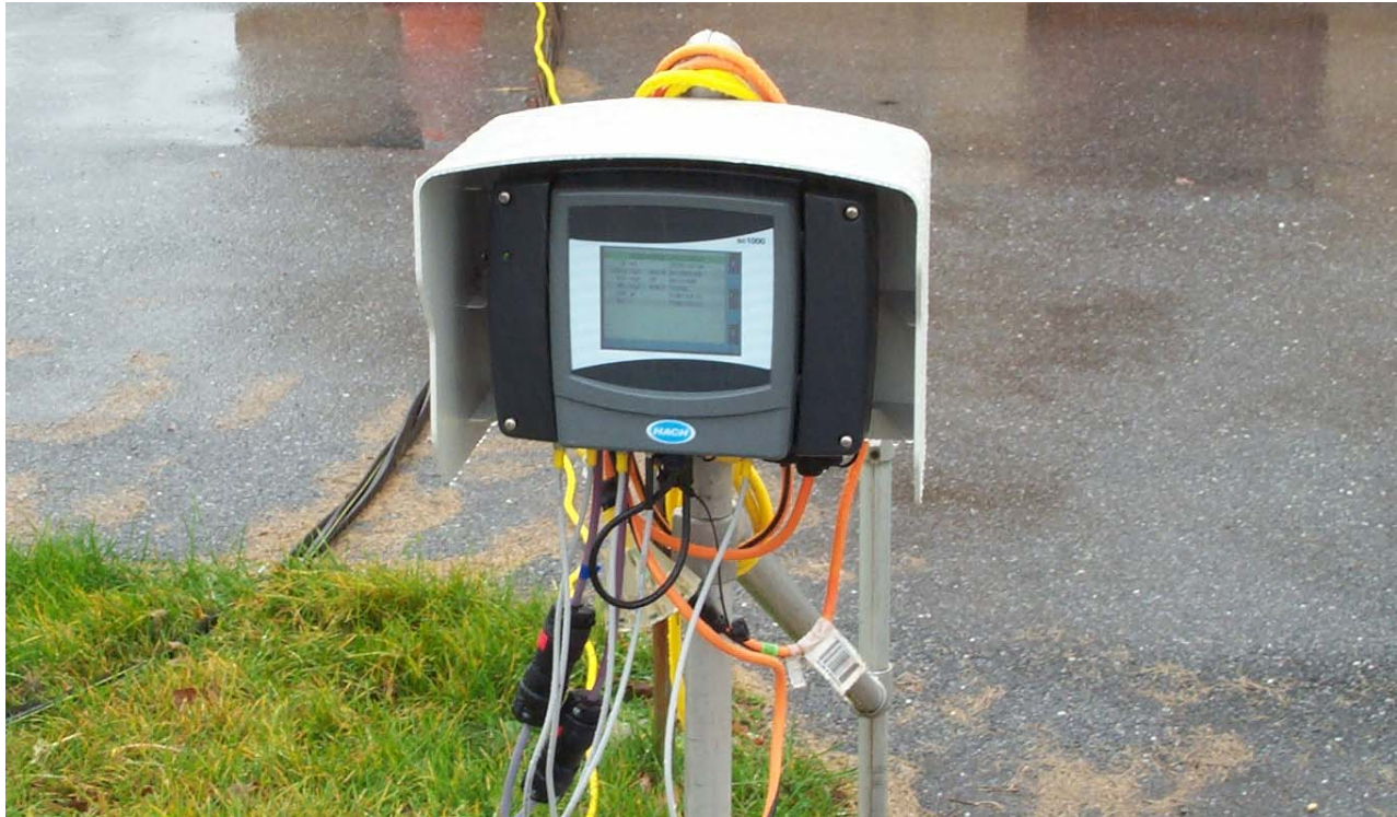
Figure F-5: Hach SC-1000 Module with Digital Display, mounted on railing near west aeration train.
