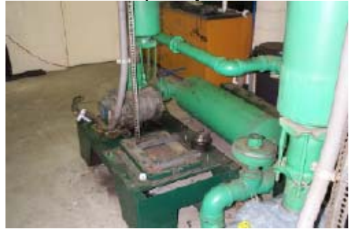
Figure: Disassembled blower system
