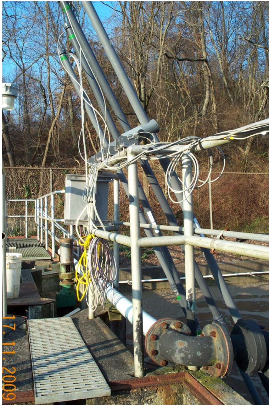
Figure 33. LDO, ORP, pH, and NH4D probes installed in east aeration tank
