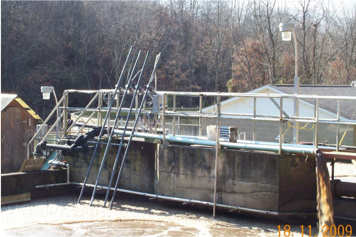
Figure 34. Nitrate, Ammonium, pH, LDO, and ORP probes installed in North aeration tank
