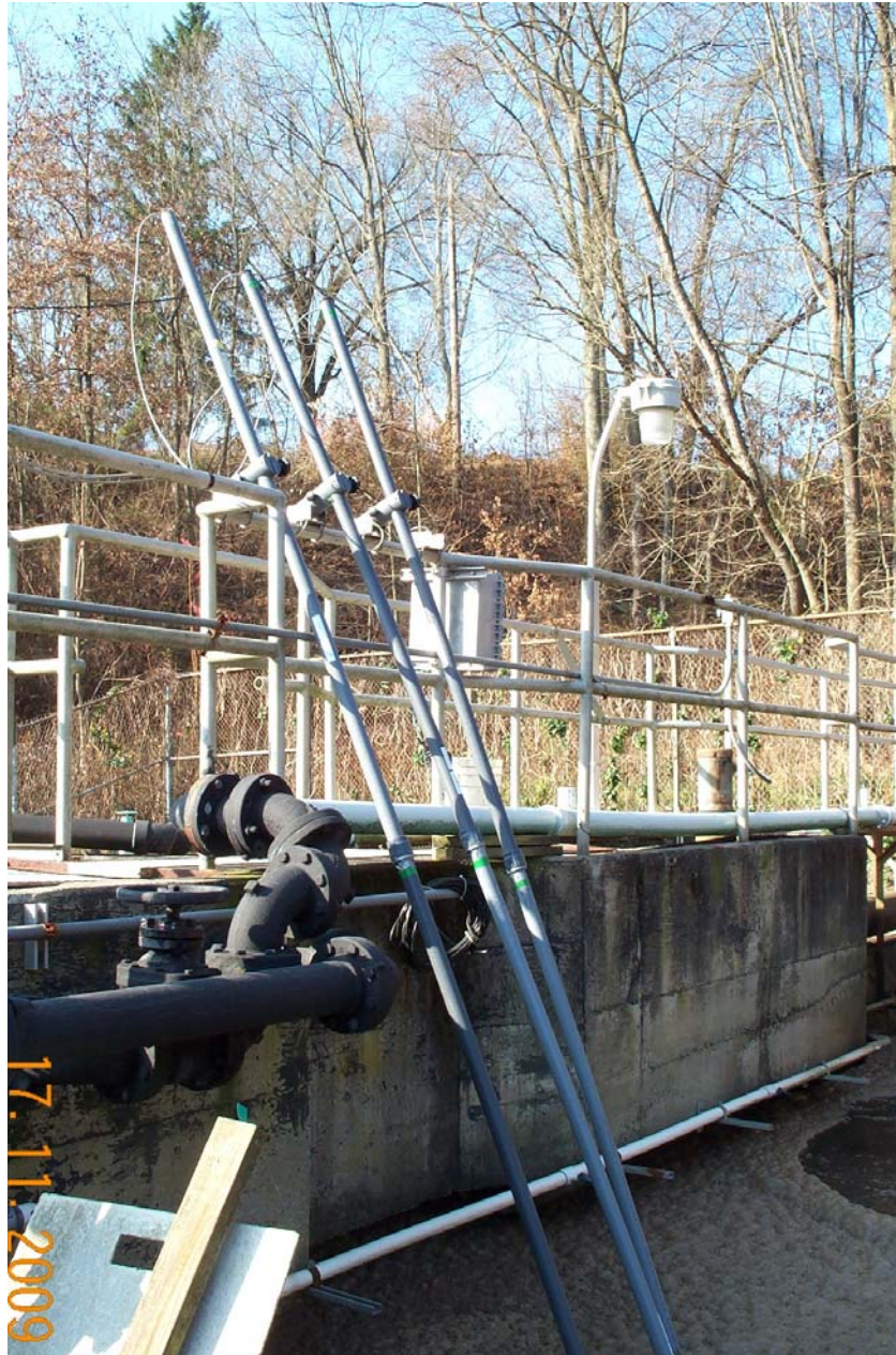
Figure 32. DO, ORP, and pH probes installed in east aeration tank
