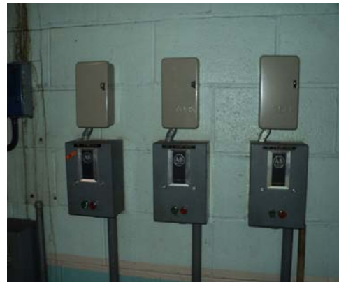
Figure G-12: Permanent installation of Blower timers, done after the evaluation.
