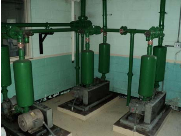
Figure G-9: PD Blowers in Control Building
