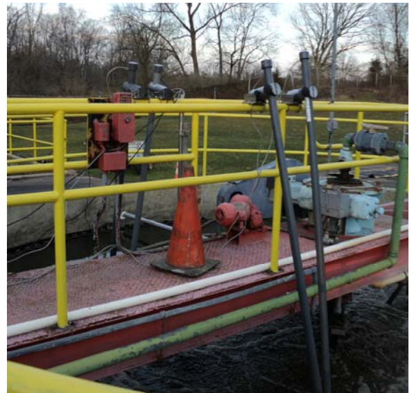
Figure G-6: Probes in Tank 3
