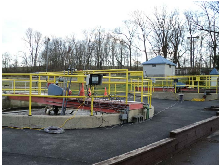
Figure G-2: View of Eimco Treatment Units with Hach SCADA equipment in place for study.
