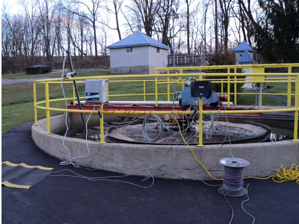
Figure G-13: Ammonia probe and controller unit in Tank 1.
