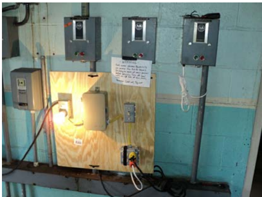
Figure G-11: Blower motor starters with timer attached.
