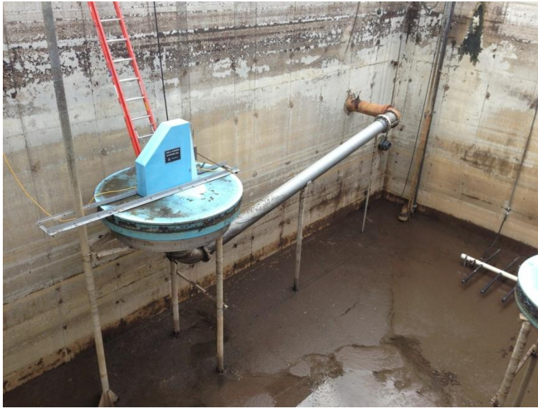
Figure 4: Decanter in SBR tank off line for maintenance
