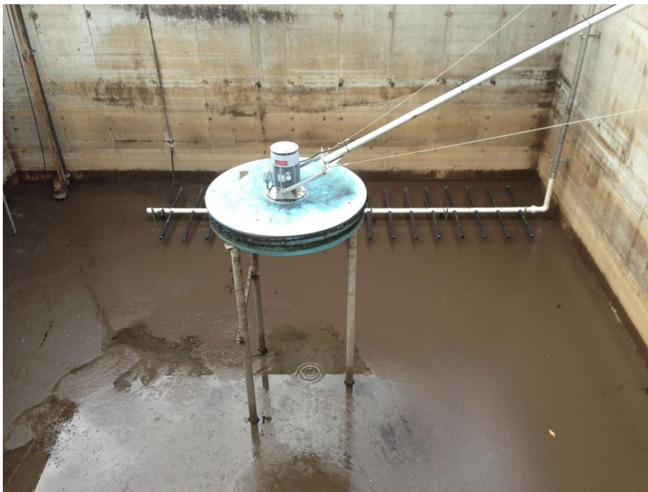
Figure 4: Mixer in SBR tank off line for maintenance
