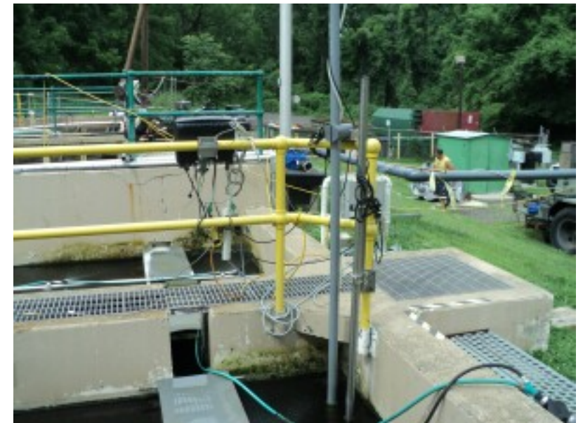
Figure 5-4: Clarifier Effluent End with WTE Probes Installed
