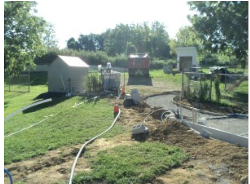
Figure 5-14: Temporary carbon feed arrangement & pump shed
