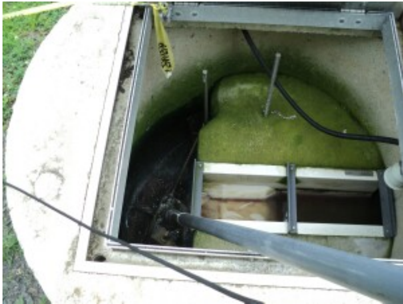
Figure 5-5: Influent Parshall Flume with BOD probe in well
