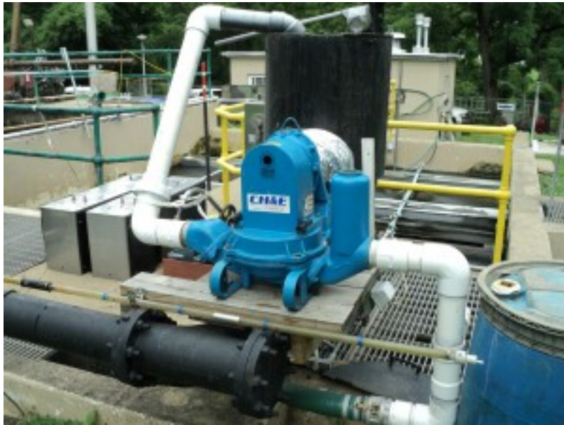
Figure 5-9: Reciprocating sludge pumps
