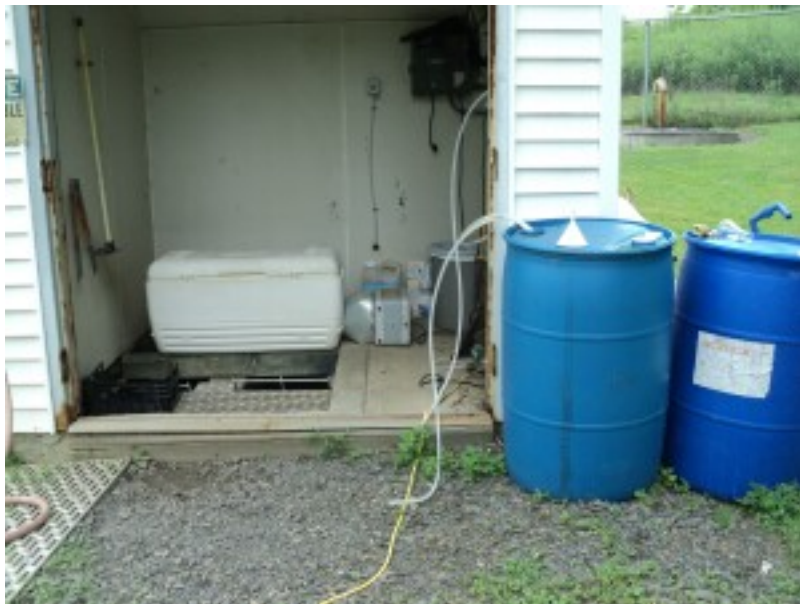
Figure 5-7: Overview of STP from former Comminutor vault
