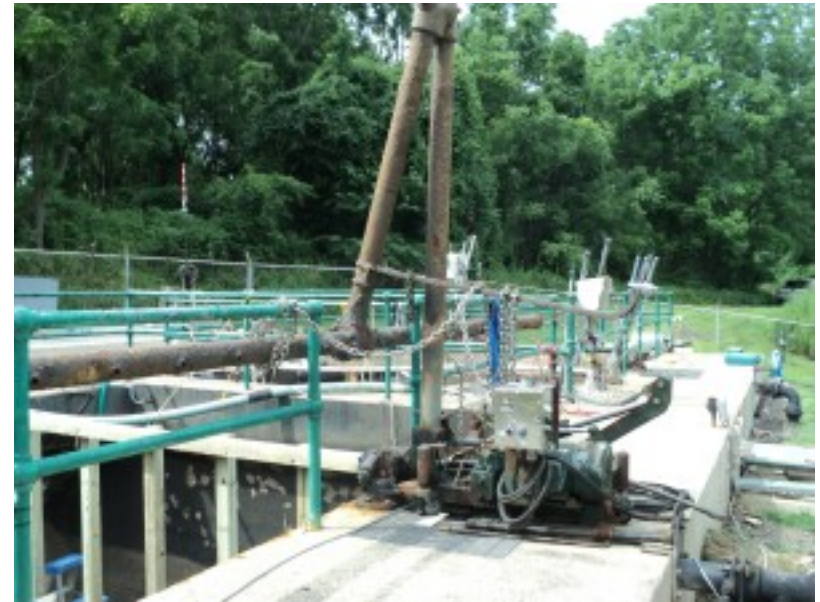
Figure 5-10: Original air header for Tank 2
