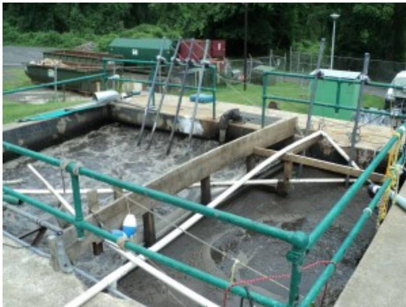
Figure 5-3: Modified MLE Tank with WTE Probes Installed
