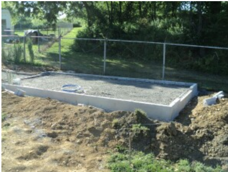
Figure 5-13: Foundation for supplemental carbon feed building
