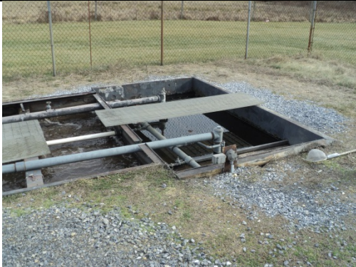
Photo 7: Clarifiers with air-lift pumps
