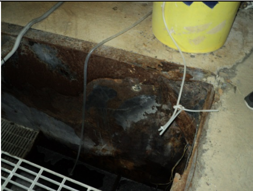
Photo 13: View of tank corrosion
