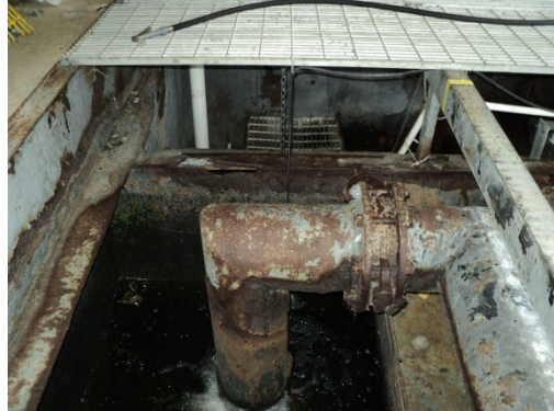
Photo 12: View of tank corrosion
