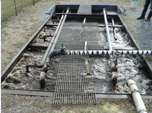
Photo 5: Secondary Treatment Unit
