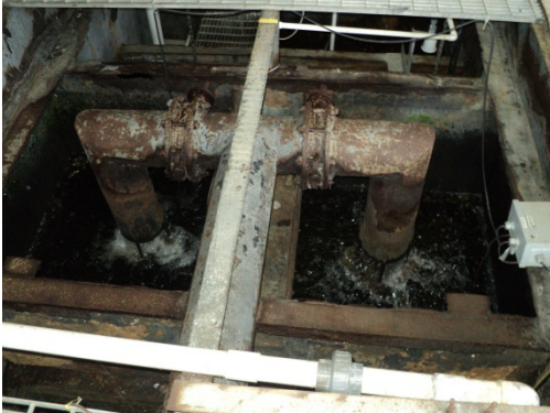
Photo 11: View of Filter Cells
