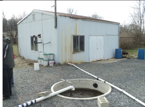
Photo 8: View of Existing Filter/Blower Building
