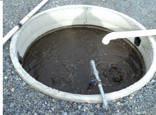
Photo 6: Sludge Holding Tank / Digester
