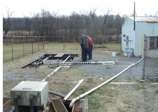
Photo 4: View from EQT to Secondary Treatment Unit
