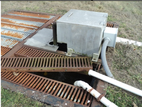
Photo 3: Equalization Tank & Inflow Lift Pumps
