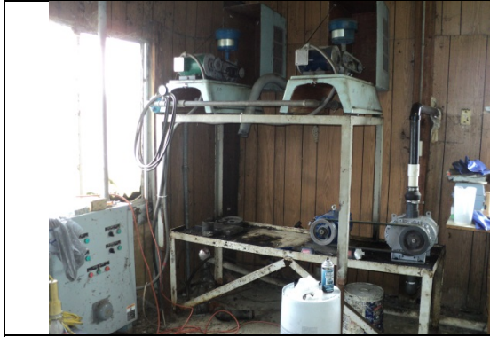
Photo 9: Air Compressors / PD Blowers
