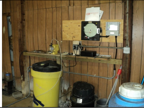
Photo 10: Disinfectant tank & Flow Meters
