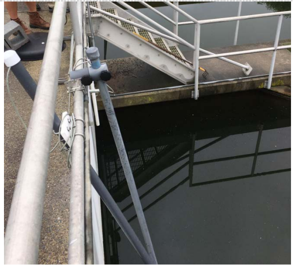
Photo 2: New ORP and Existing DO probes
