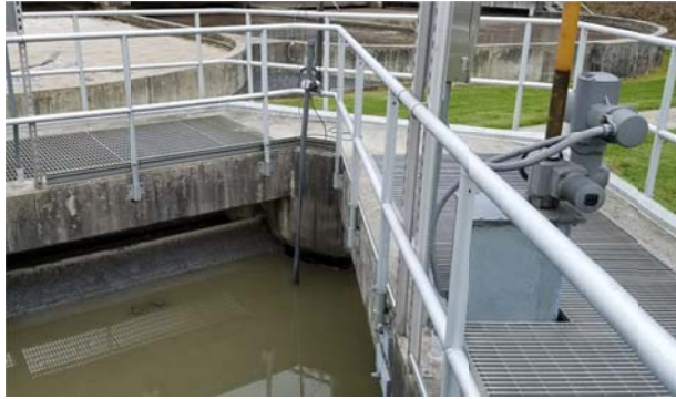
Photo 1: TOC probe at Influent Splitter
