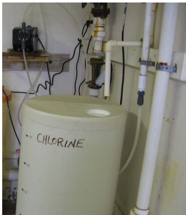
Chlorine system picture:
