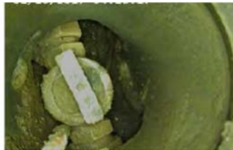
Non-Lead Service Line
