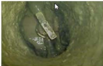
Lead Service Line
