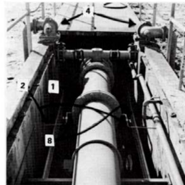
Air distribution piping in the Y-wall of a large activated sludge plant connected to air headers.
