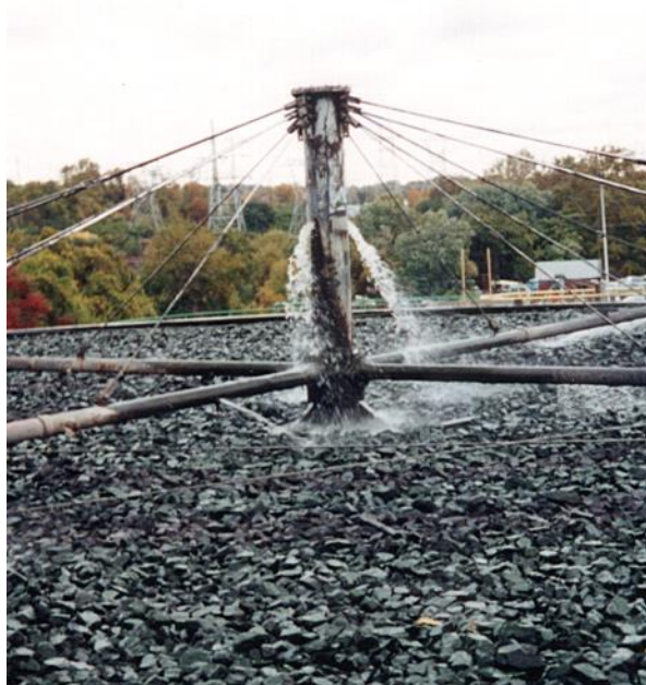
Figure 3.1 Tickling Filter with Leaking Seals
