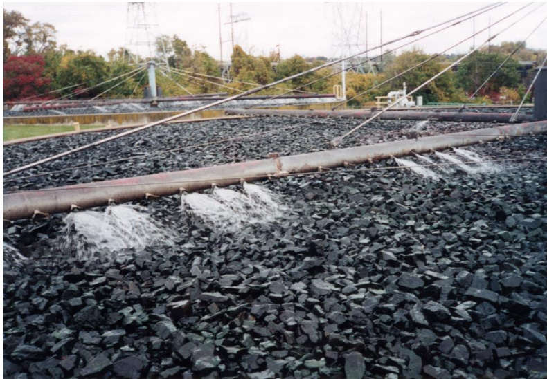
Figure 3.2 Tickling Filter with Clogged Nozzles
