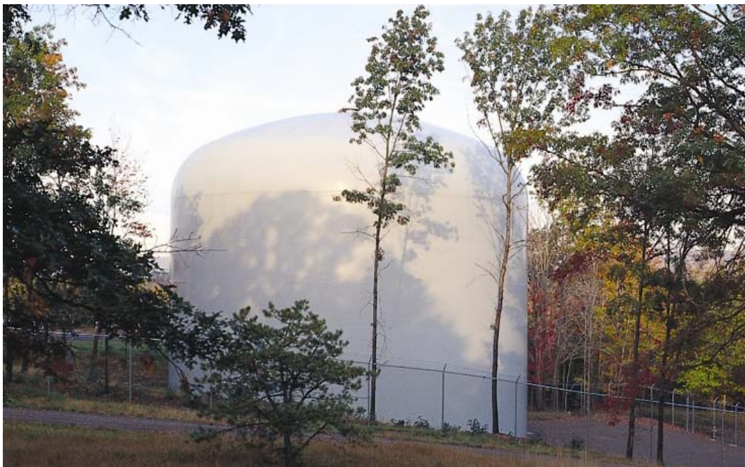
Figure 3.2 – Ground Level Tank
