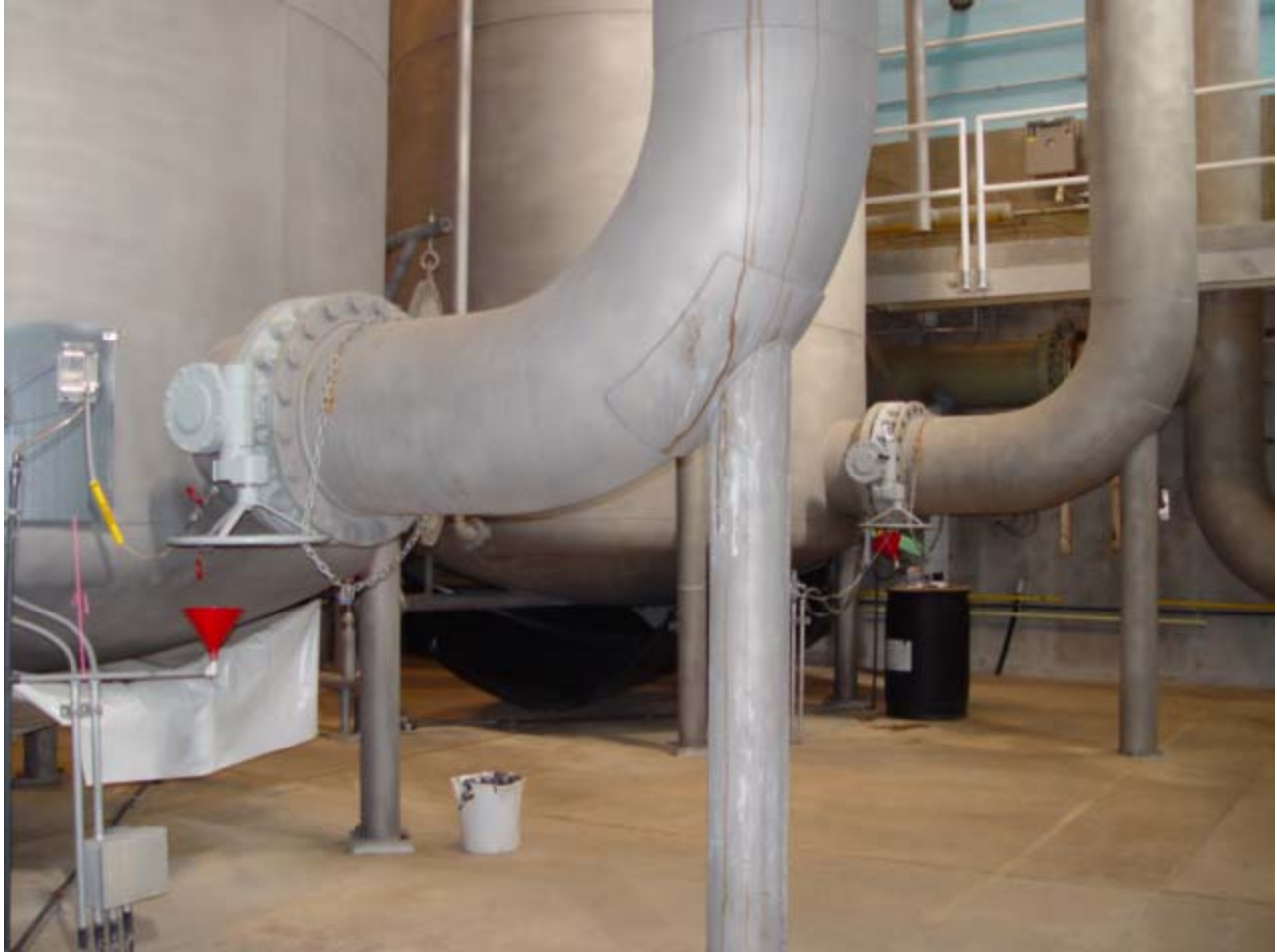
Figure 4.5 Stainless Steel Piping Showing Evidence of MIB Pinholes
