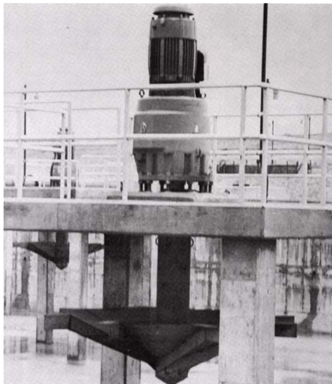
Figure 2.1 Mechanical Aeration Device 1
