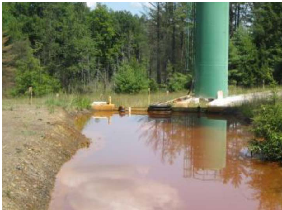
Tipping bucket lime doser treating AMD Discharge No. 17 PA 1934
