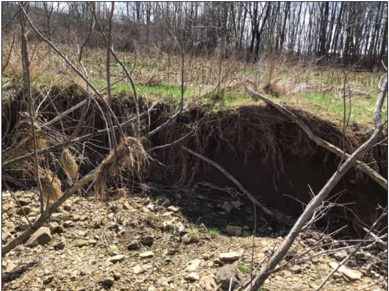
photo 15: Streambank erosion along an unnamed tributary to Evitts Creek.
