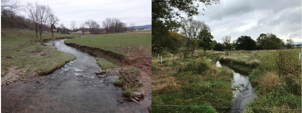
Figure 10: Before (2018) and after (2020) installation of fencing, crossing, and buffer planting at upstream end of Weaver Martin farm, Susqueheca Creek.
