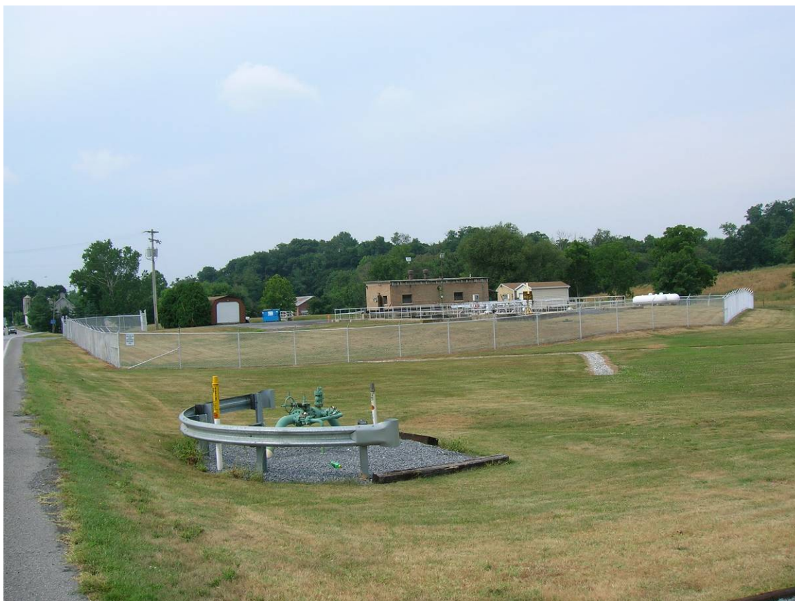
Above – Sewage Treatment Plant along Rte. 997
