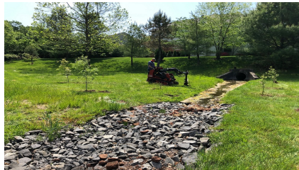
Figure 2: Channel Construction- Removal of the entire eastern low flow channel and selected sections of the southern low flow channel. Removed sections were replaced with filter fabric and stone to allow for infiltration and to disperse stormwater.
