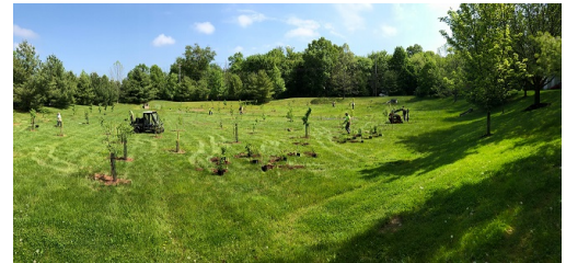
Figure 3: Basin Planting- Following several months of monitoring after channel removal, 150 native trees, shrubs and a meadow were planted in late spring.
